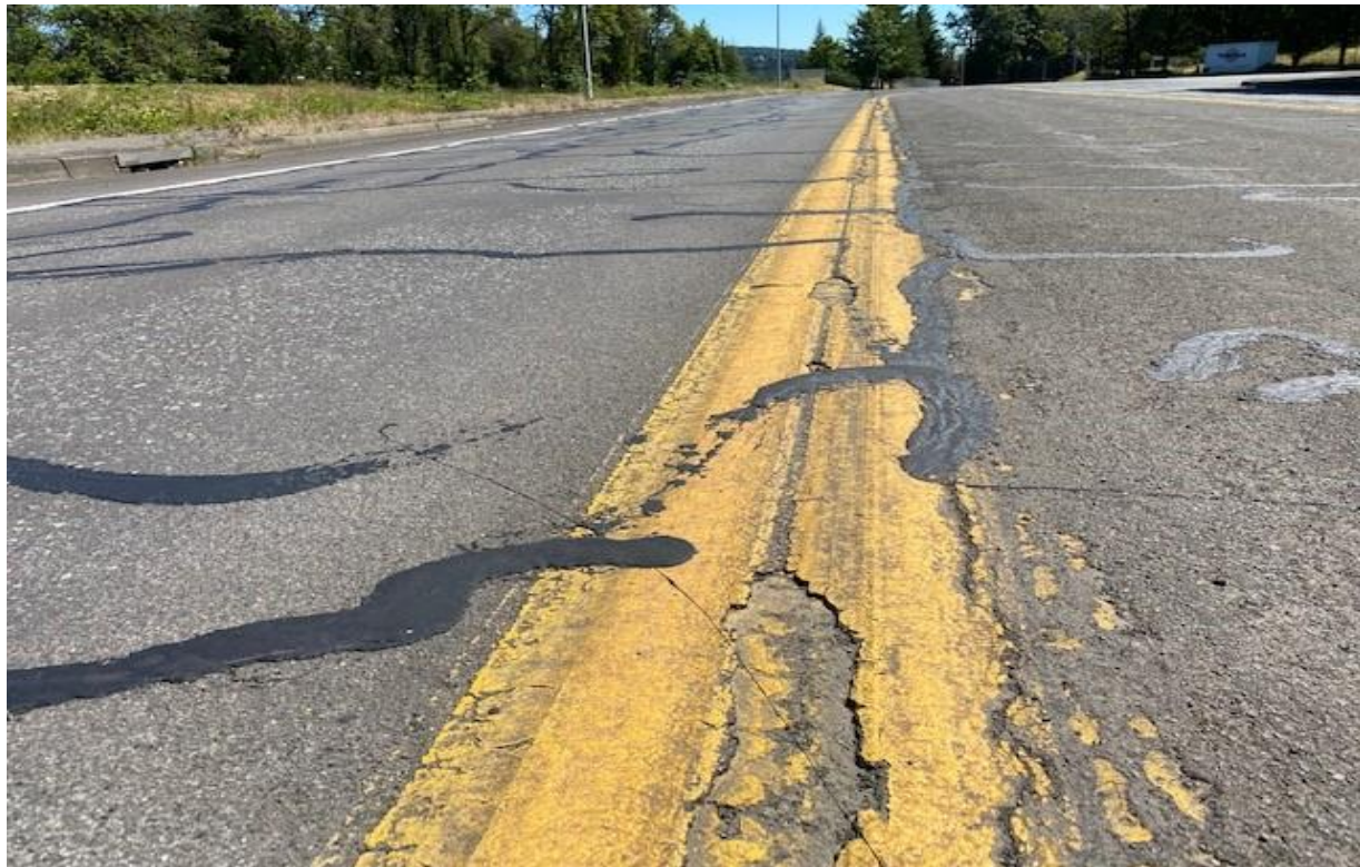
NW Parker Looking South towards WaferTech: Layers of existing street markings were delaminating from the pavement surface.
