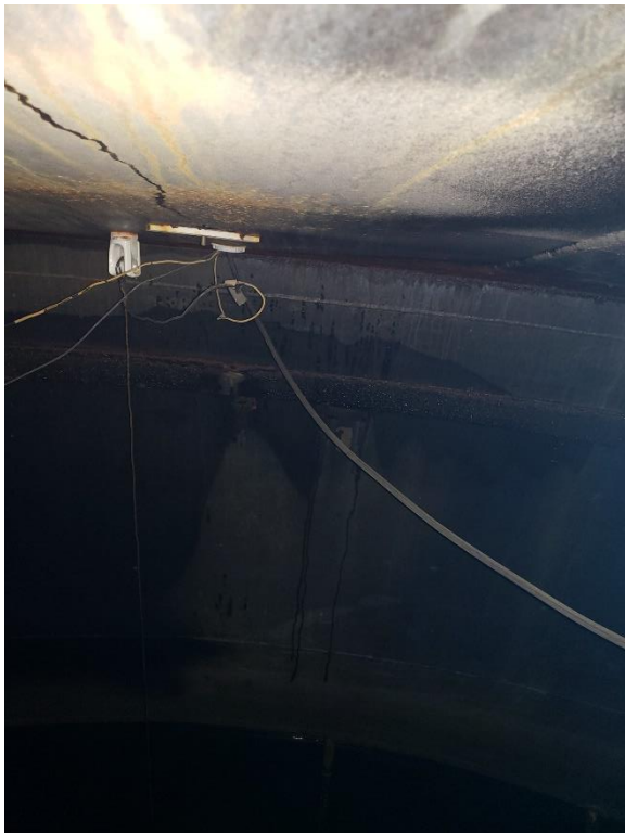
It appeared they may be an internal platform, though difficult to make out.
