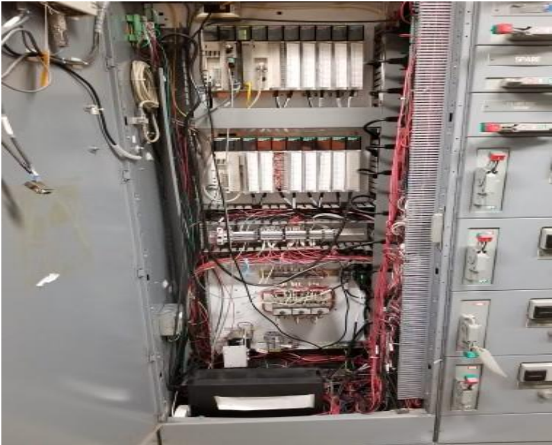
Figure 1: Existing PLC with wiring modifications over time
