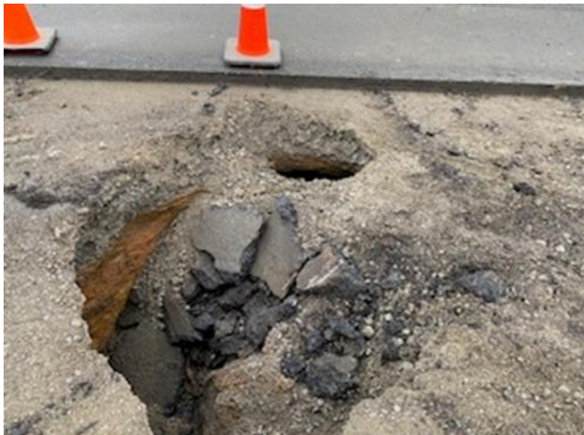
Figure 1. Sinkhole under Endicott St.
