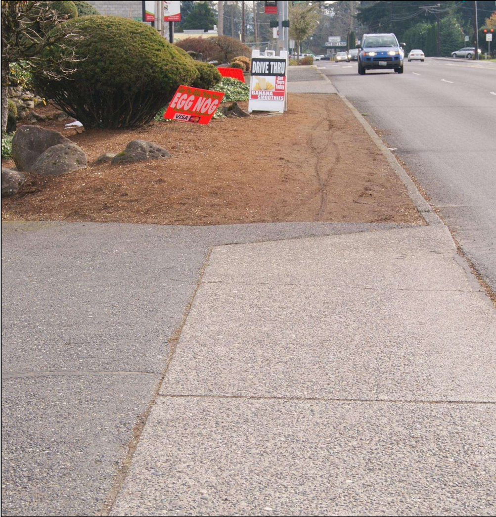
Figure 6: Examples of existing missing sidewalk section
