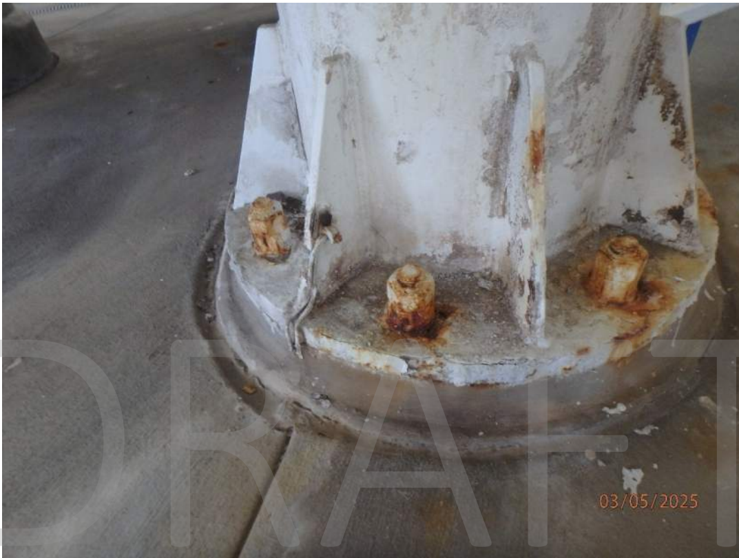
Figure 4: Typical Corrosion at Foundation Anchors
