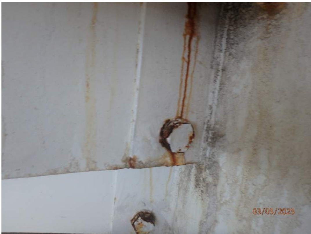
Figure 9: Heavy Corrosion of Bolt at Central Column
