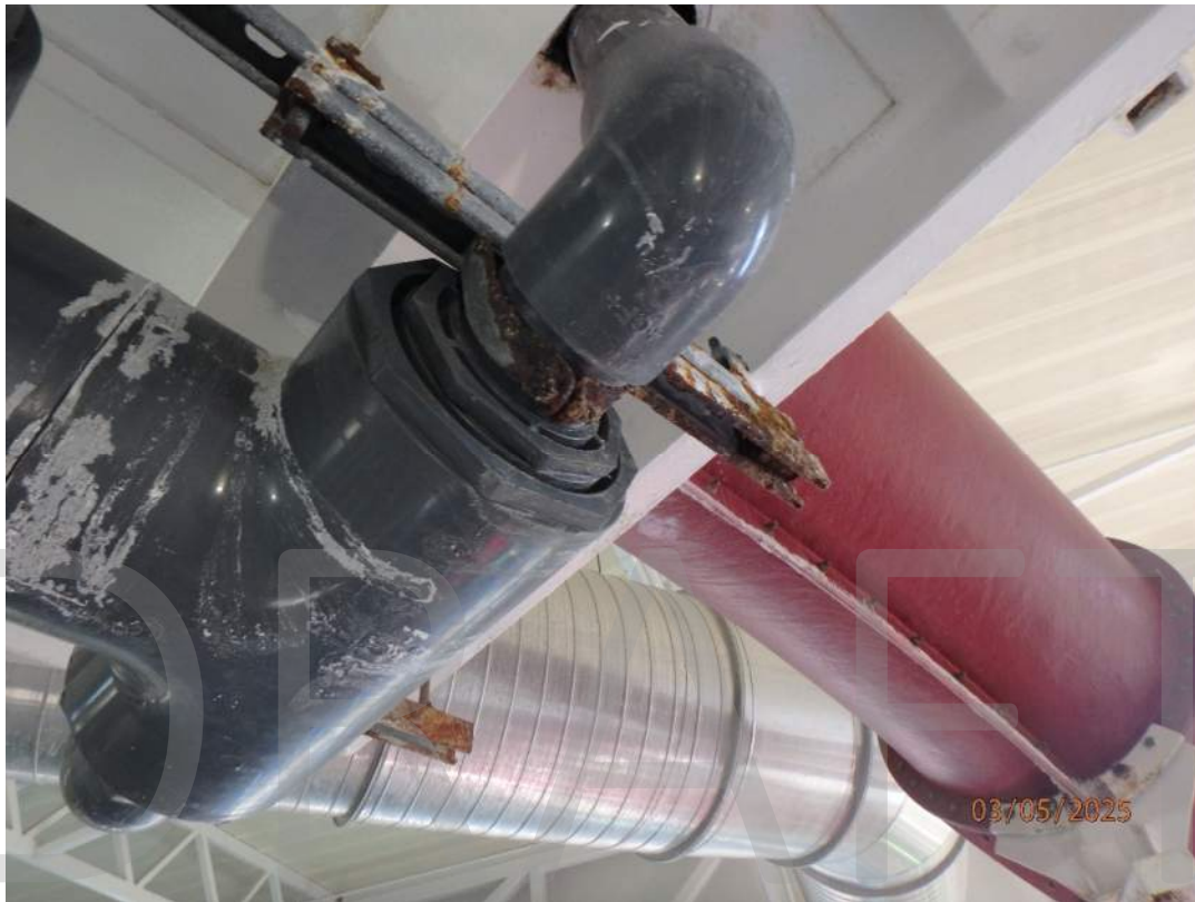
Figure 8: Typical Heavy Corrosion at Pipe Supports below Upper Platform
