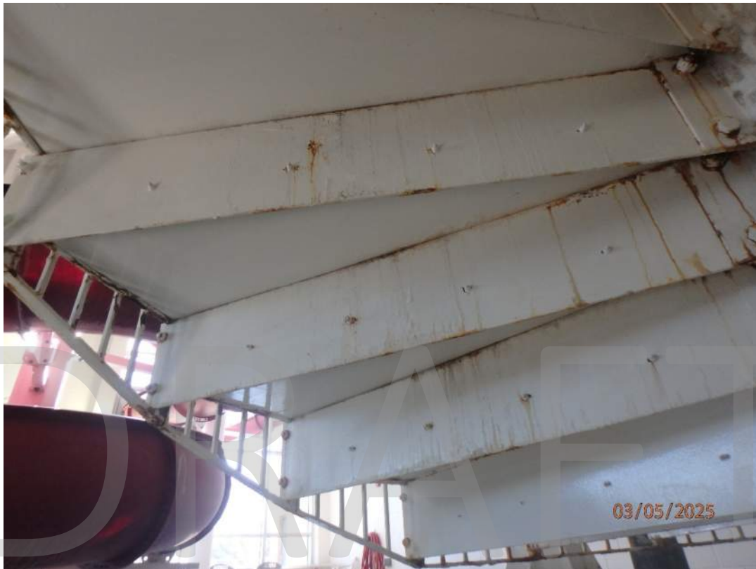
Figure 2: Typical Corrosion Stains at Back of Risers
