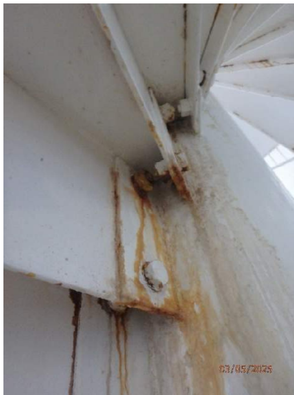
Figure 3: Typical Corrosion of Bolts at Central Support Column
