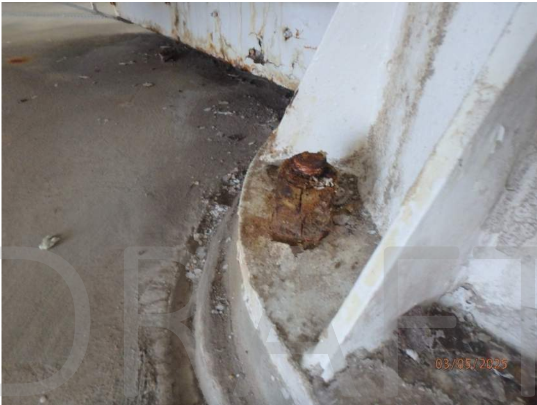
Figure 10: Heavy Corrosion at Foundation Anchors
