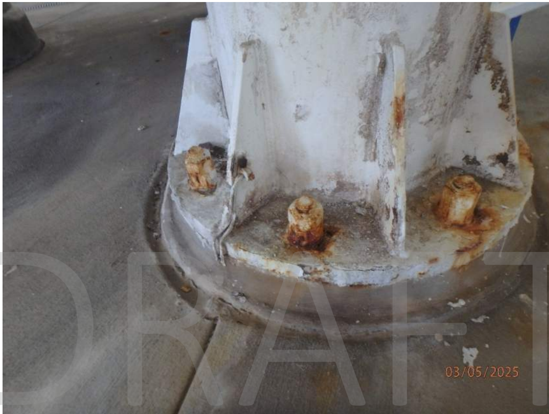
Figure 4: Typical Corrosion at Foundation Anchors
