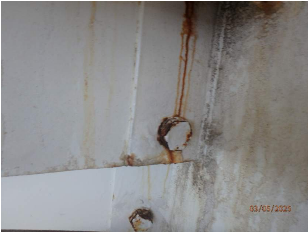
Figure 9: Heavy Corrosion of Bolt at Central Column
