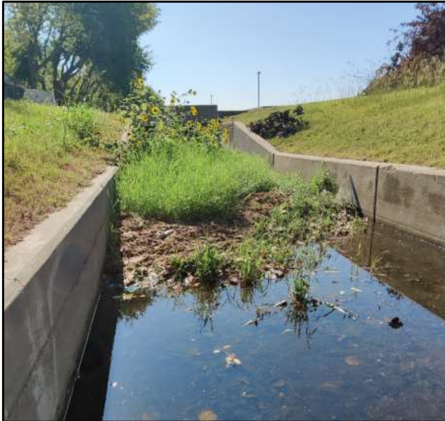
Clogged drainage along SW Murphy
