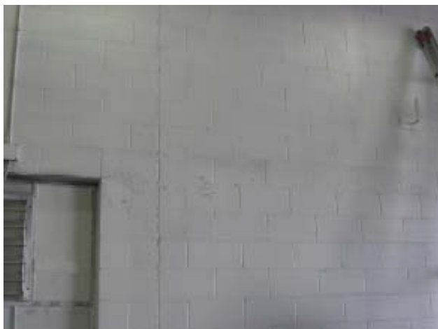
Fig 82: Garage - Vertical masonry crack in expansion joint on both interior and exterior surfaces of west wall
