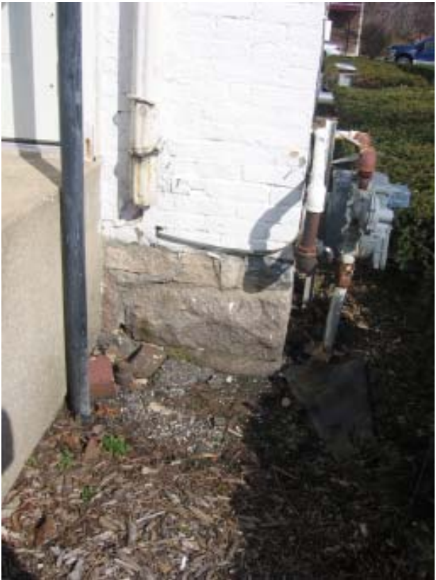
Fig 9: East elevation - Downspout discharging directly against foundation
