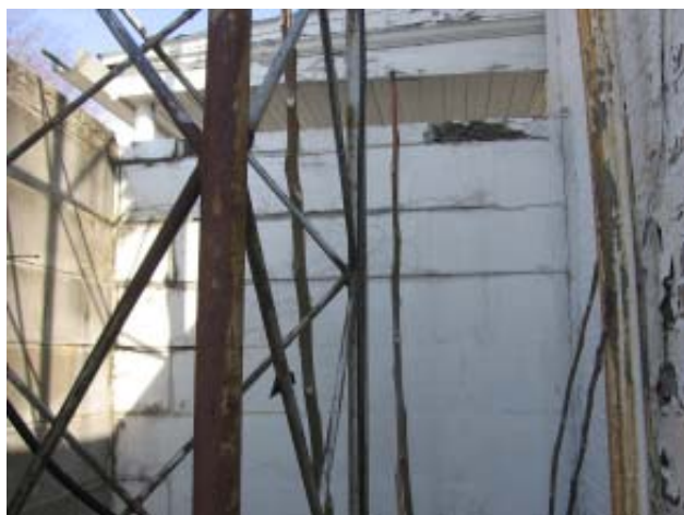
Fig 23: West elevation - Deterioration of top courses of antenna enclosure cmu walls
