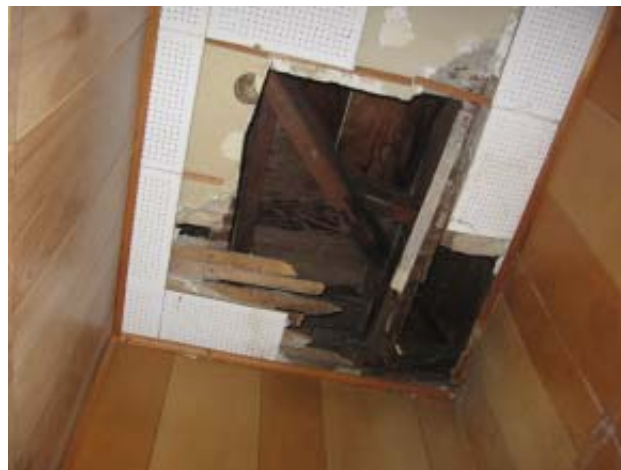
Fig 54: Attic and Roof Structures- Water staining in southeast corner of the east wing
