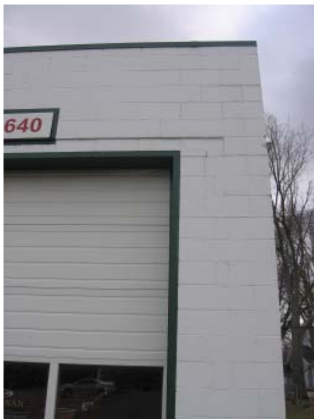
Fig 68: Garage- North elevation, step cracking at lintel bearing and western corner of wall
