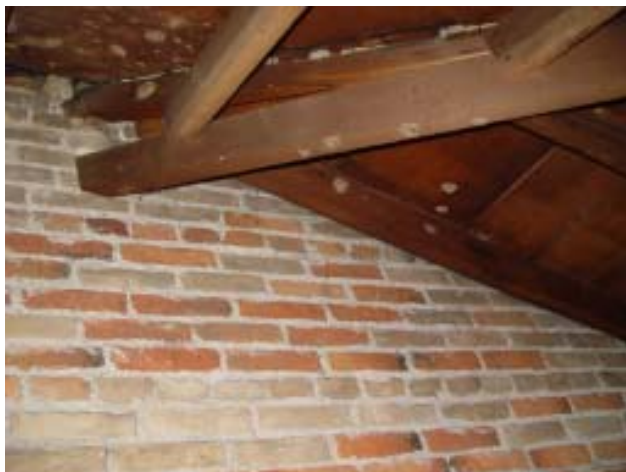
Fig 56: Attic and Roof Structures- Severely split hip ridge member at wall bearing, west wing
