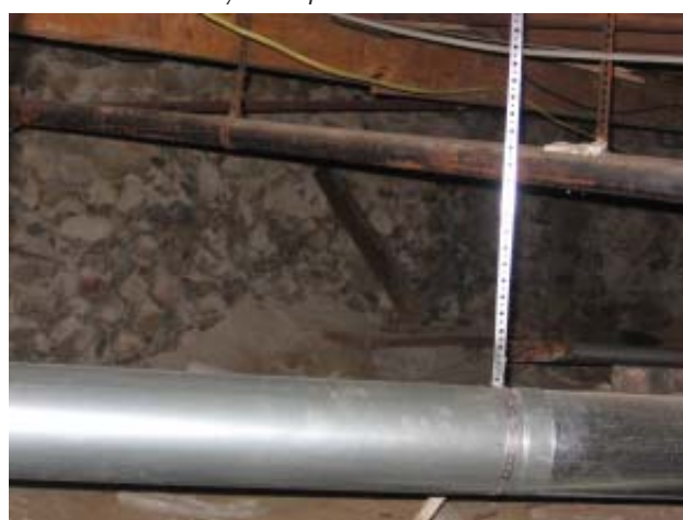
Fig 35: East Crawl Space - Wood bracing system along east exterior wall, excessive mortar dust pile
