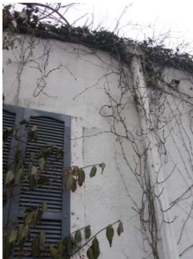
Fig 69: Garage- East elevation, heavy vegetation growth in gutter system
