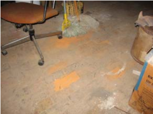
Fig 28: Basement - Deteriorated floor pavers
