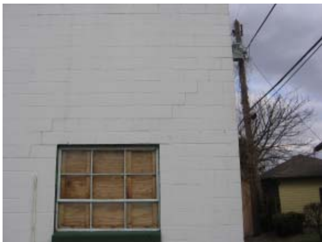
Fig 75: Garage- South elevation, step cracking south of southern window
