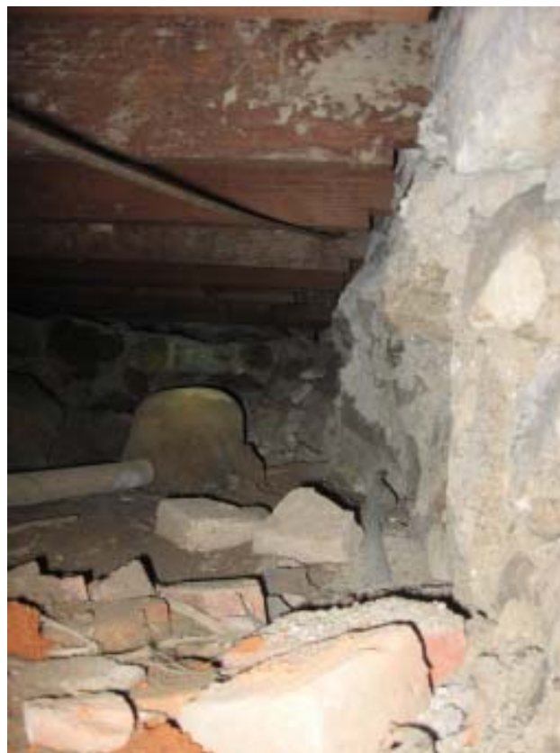
Fig 45: First Floor Structure - Notched joists at east bearing in west wing
