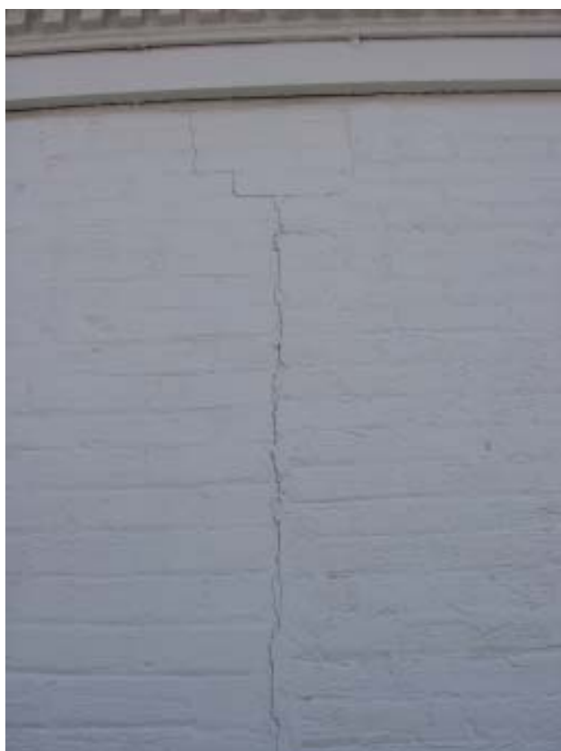
Fig 27: West elevation - Vertical crack at construction joint
