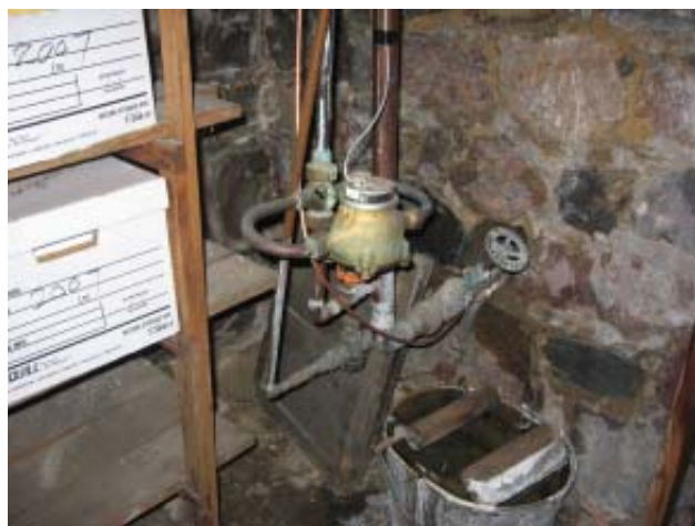
Fig 32: Basement - Leak near a utility meter captured into overflowing bucket below
