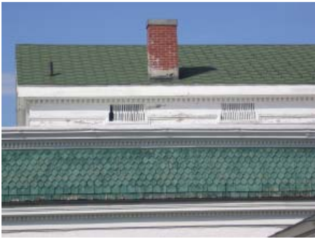
Fig 10: East elevation - Missing iron bar
