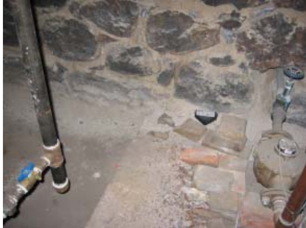
Fig 31: Basement - Mortar dust at base of south wall
