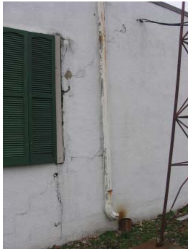
Fig 71: Garage- East elevation, downspout discharging against exterior wall and step cracking in masonry
