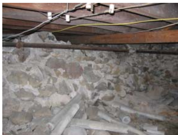
Fig 34: East Crawl Space - Stone masonry walls, excessive masonry dust presumed asbestos insulation
