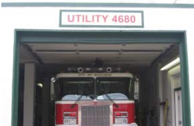
Fig 66: Garage- North elevation, visual sag in lintel
