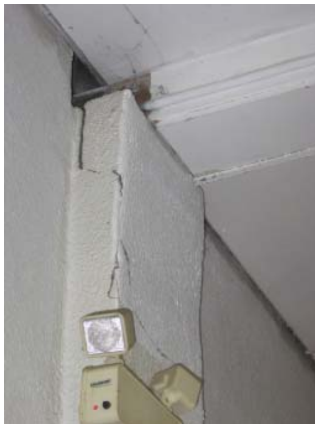
Fig 78: Garage - Masonry pier for roof beam bearing is cracked and rotating inward
