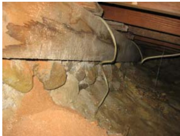
Fig 38: West Crawl Space - Excessive brick masonry dust at base of walls; loose stones in foundation wall
