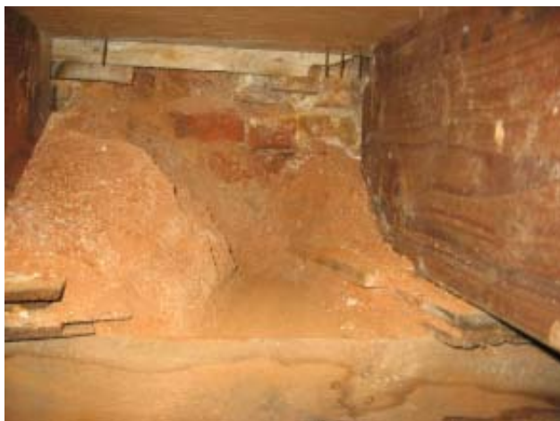
Fig 36: West Crawl Space - Excessive brick masonry dust at base of walls
