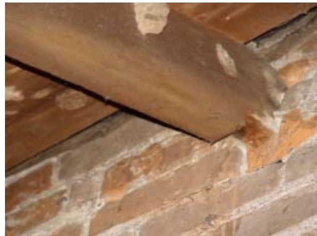
Fig 57: Attic and Roof Structures- Significant movement of rafters out of bearing pockets in west wing
