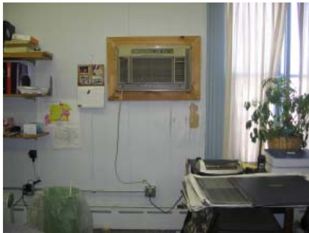
Fig 47: First Floor Level - Water damage below air conditioning unit in east exterior wall
