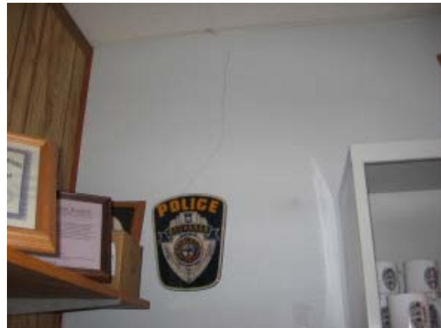
Fig 49: First Floor Level - Crack in west wall, north end of west wing
