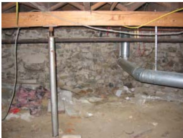
Fig 44: First Floor Structure - Visual curvature in center beam in east wing
