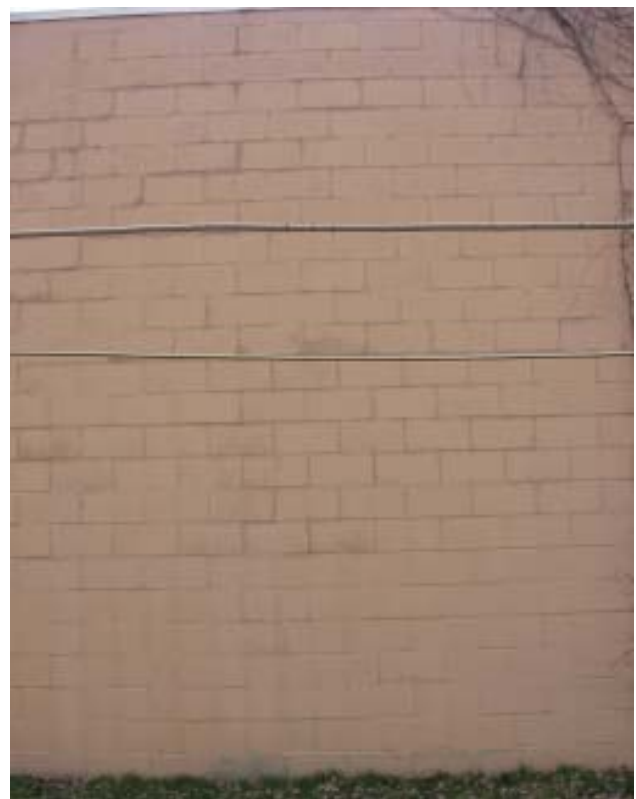
Fig 74: Garage- South elevation, south wall of addition cracking and moisture shown
