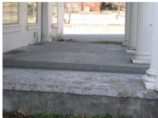
Fig 5: Concrete slab of north porch
