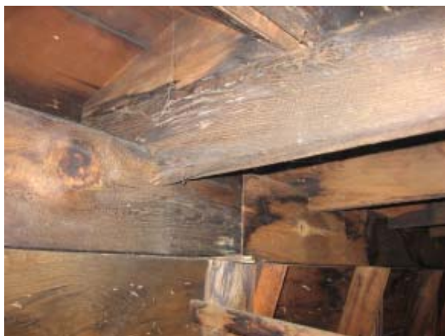
Fig 63: Attic and Roof Structures- Extensive water damage at mansard wall framing in west wing
