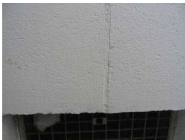
Fig 21: South elevation - Cracked cmu over vent
