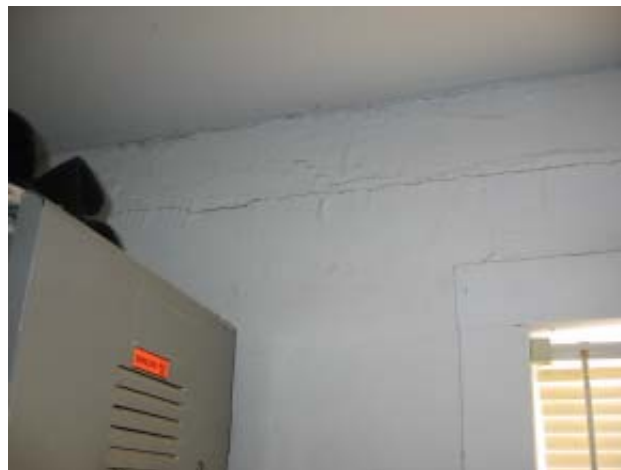
Fig 51: First Floor Level - Horizontal crack at top of jail west wall
