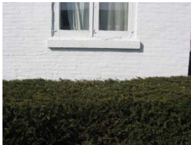
Fig 8: East elevation - Cracking below window
