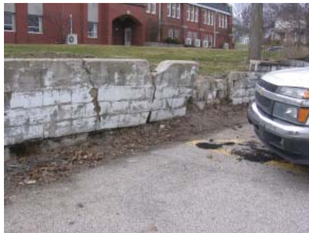
Fig 77: Failing retaining wall at west edge of property
