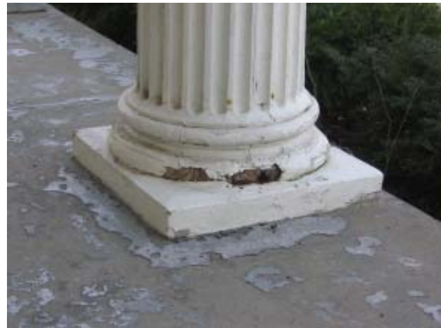
Fig 4: Deteriorating column bases at north porch
