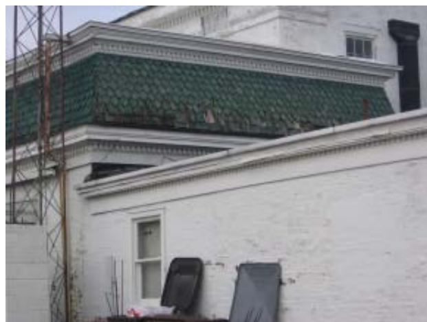
Fig 20: South elevation - Deteriorated shingles
