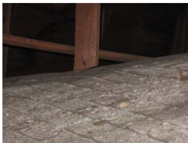
Fig 61: Attic and Roof Structures- Gap observed between bottom of stud supporting hip ridge and top of original hipped roof in west wing
