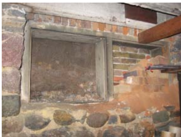
Fig 33: Basement - Window infill and deteriorating brick at north wall
