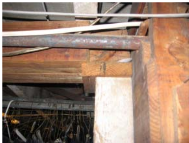
Fig 39: First Floor Structure - East beam line, south end, 3 of 4 plies have bearing on wood column
