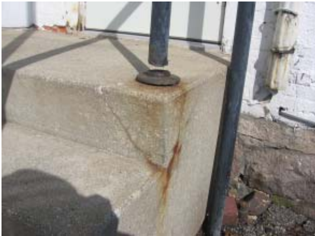
Fig 11: East elevation - Handrail support with no bearing
