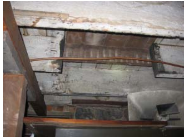
Fig 42: First Floor Structure - Cut joist in northeast corner
