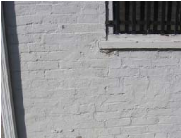
Fig 12: East elevation - Mainly vertical step crack
