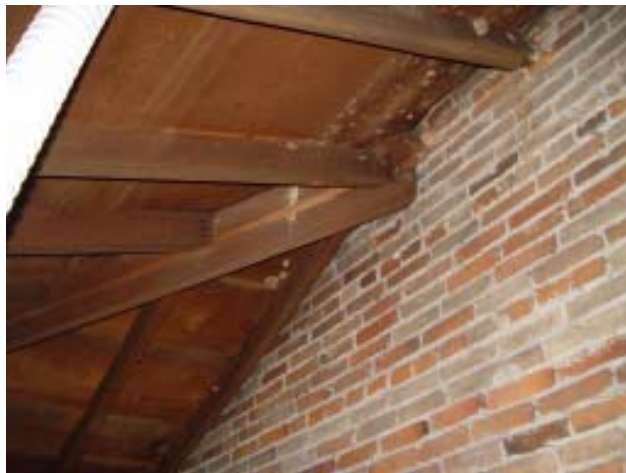
Fig 55: Attic and Roof Structures- Severely split hip ridge member at wall bearing, west wing
