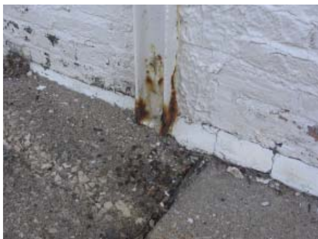
Fig 26: West elevation - Existing channel brace rusting
