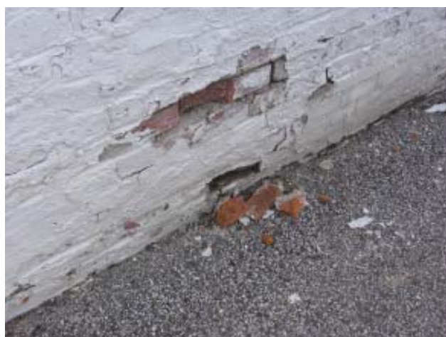
Fig 22: West elevation - Severely deteriorated brick
