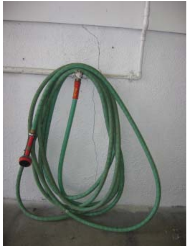
Fig 80: Garage - Vertical masonry crack in common wall between original and addition buildings
