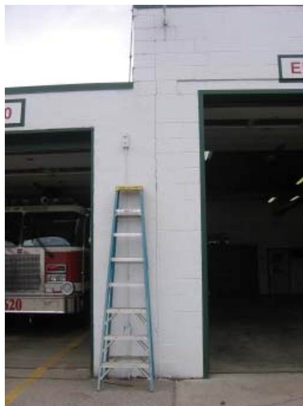
Fig 67: Garage- North elevation, vertical crack at joint between original and addition constructions
