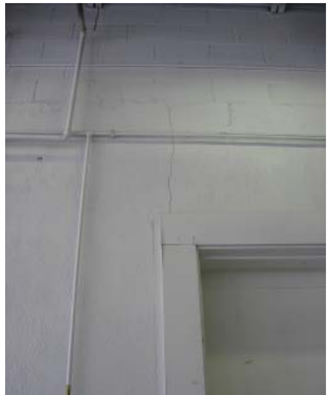
Fig 81: Garage - Vertical masonry crack in common wall between original and addition buildings; note stucco is discontinuous at new addition wall coursing
