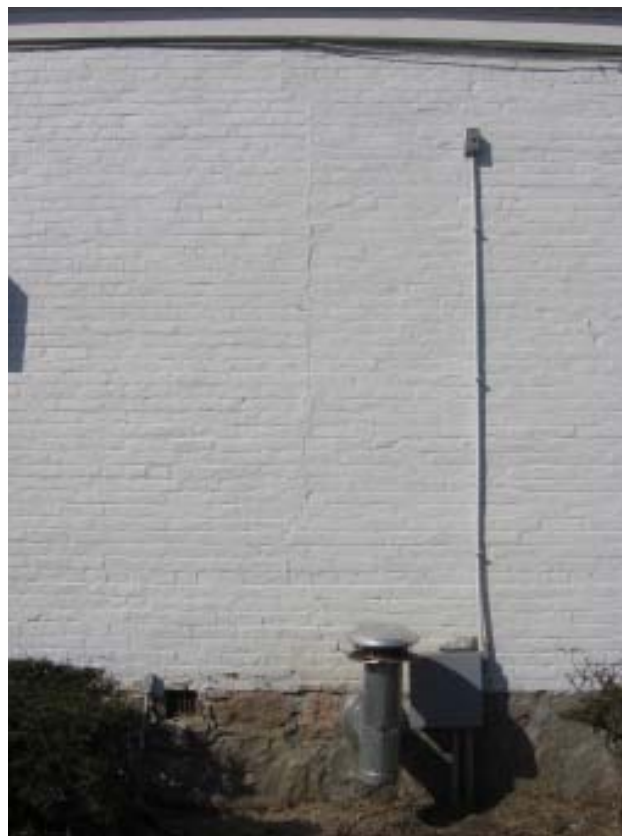
Fig 7: East elevation - Vertical cracked joint
