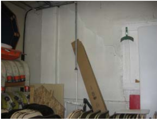
Fig 79: Garage - Masonry cracking on interior that relates to cracking on east exterior wall
