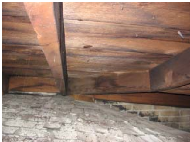
Fig 62: Attic and Roof Structures- Ledger board at masonry wall supporting rafters in west wing
