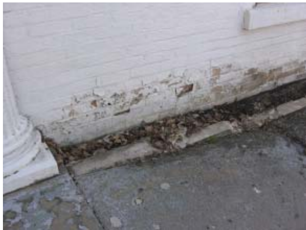
Fig 3: Deteriorating exterior brick north wall west wing
