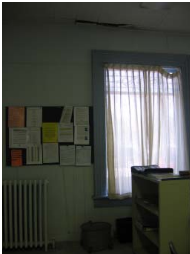
Fig 48: First Floor Level - Water damage at north wall of the east wing
