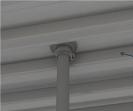
Plumbing connection under the upper basin
