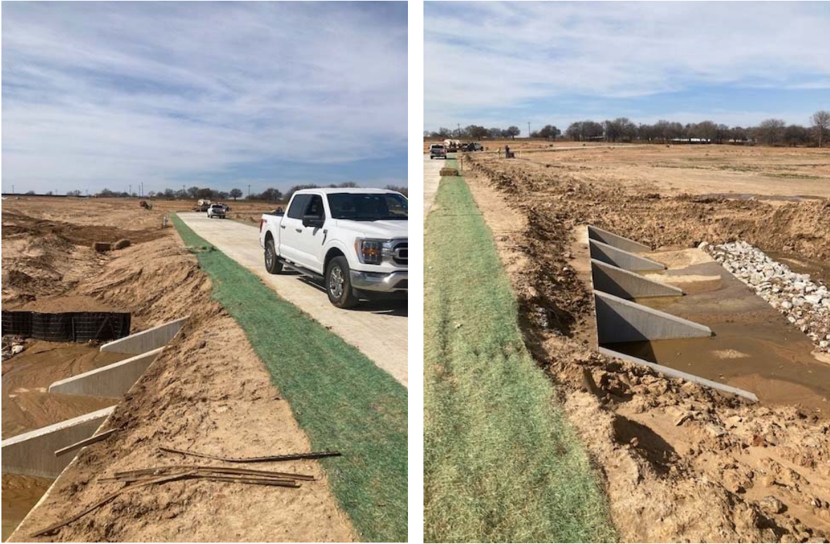
March 7, 2023 more areas that have erosion issues
