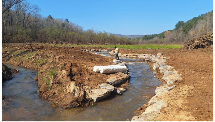
MUDDY CREEK STRUCTURE TRASH RACK MCDOWELL COUNTY, NC
