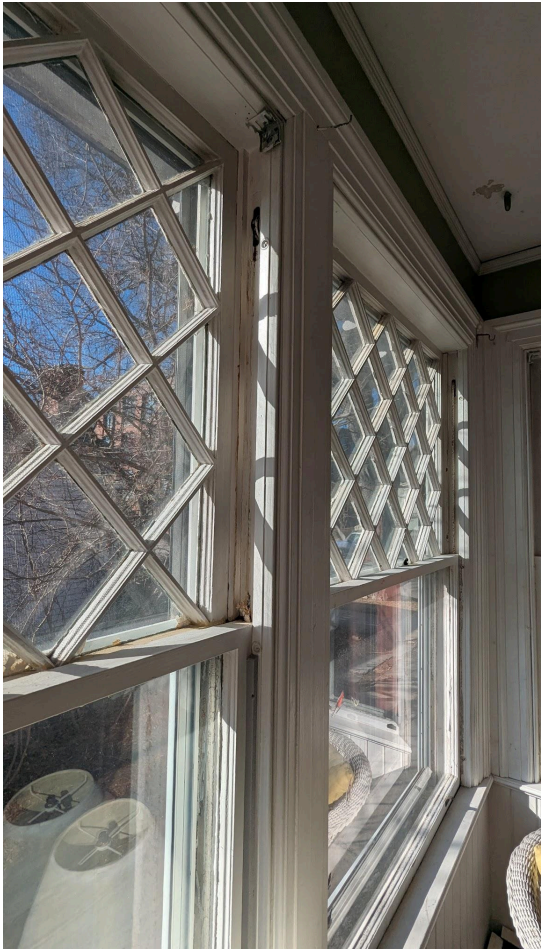
Missing sash cords
