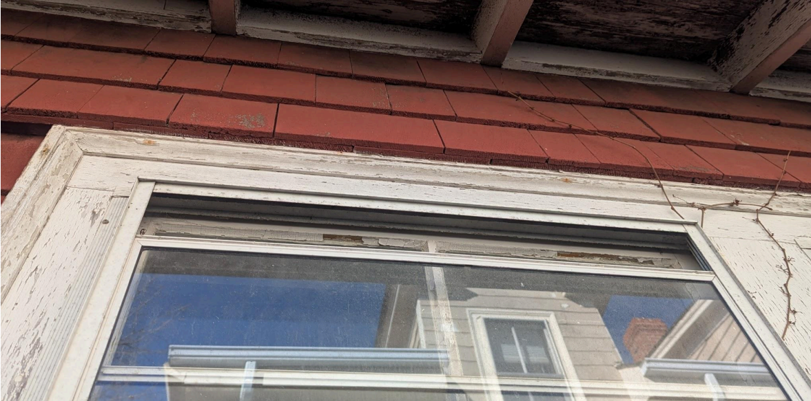
Cracked/missing glazing compound
