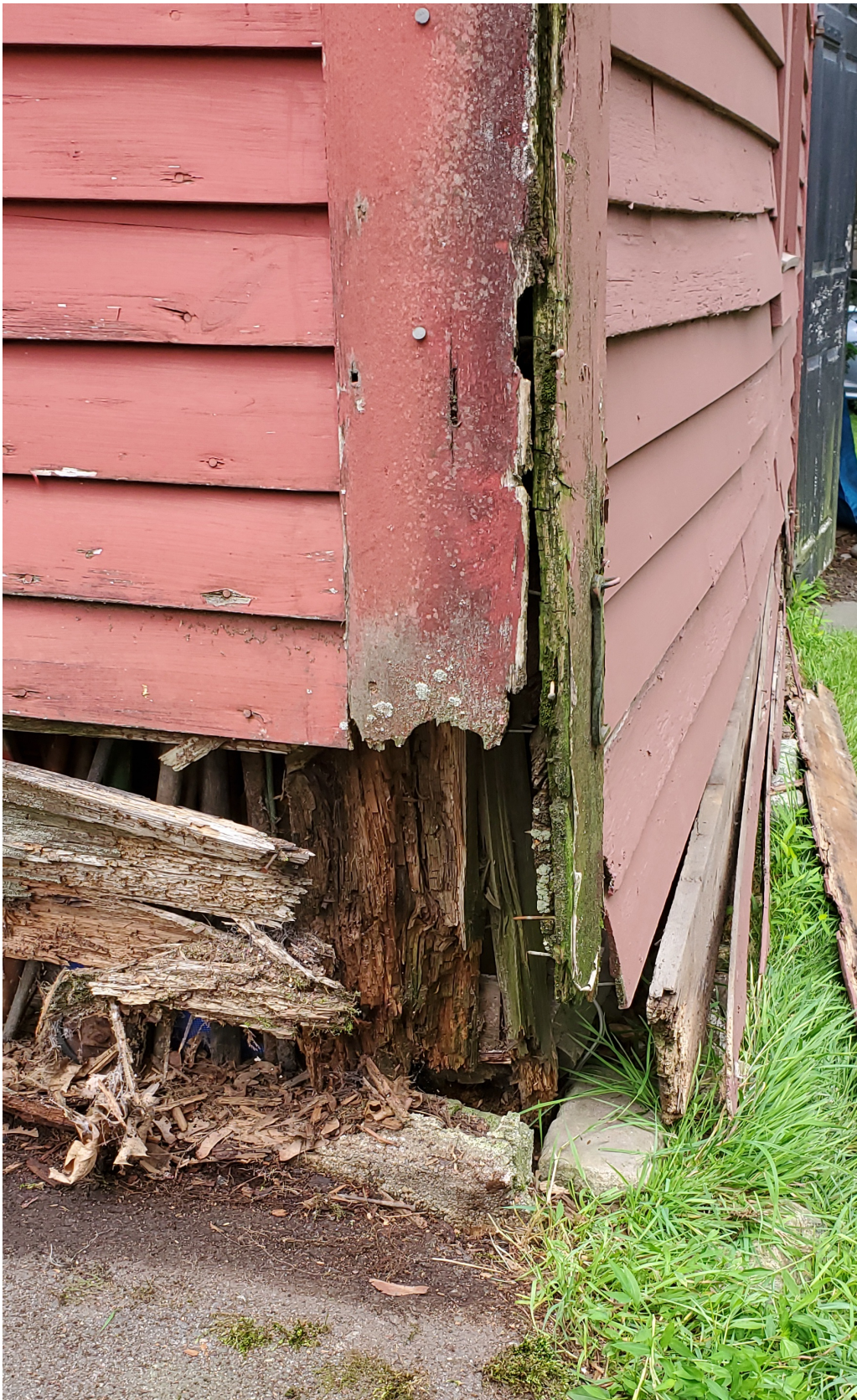
Figure 7: Corner post showing extensive rot from being in contact with rotted sill beam and ground.
