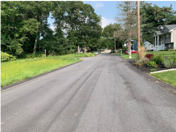
Photo No. 5: Roadway condition
