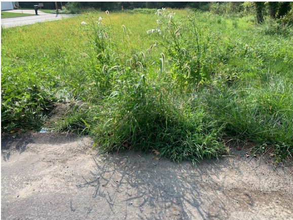
Photo No. 7: Vegetative growth within PWW
