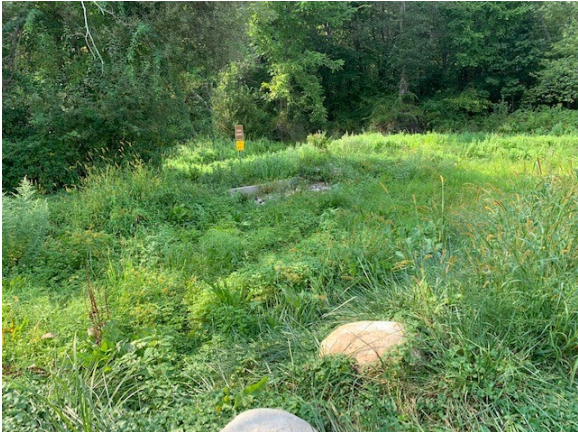
Photo No. 1: Vegetative growth within Spillway
