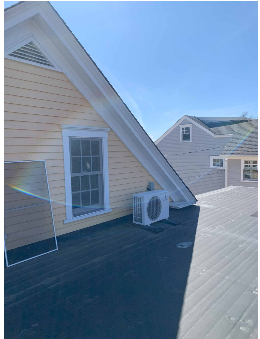
Photo #7: View of second floor condenser unit located on flat roof at rear of the home
