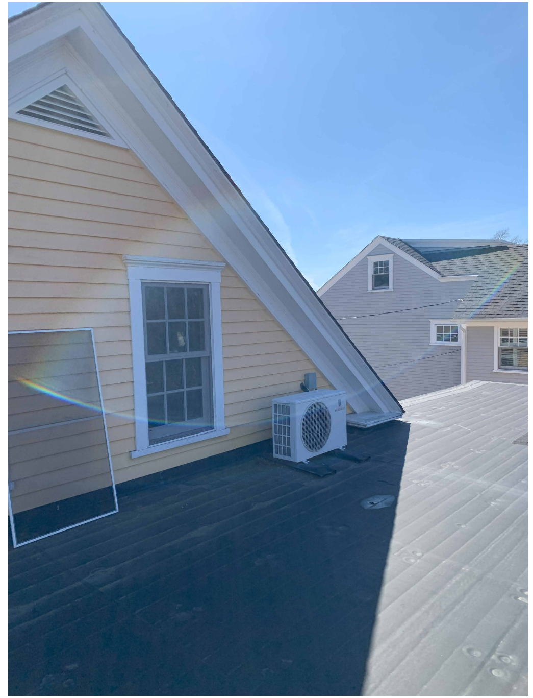
Photo #7: View of second floor condenser unit located on flat roof at rear of the home
