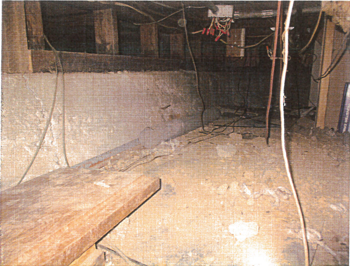
Photo 2: View within the foundation crawl space. Note the diagonal crack in the continuous interior footing near the left side of the photo.
