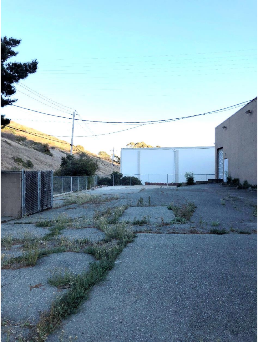
View of rear yard and parking lot looking east. 150 W. Hill Pl. in background.
