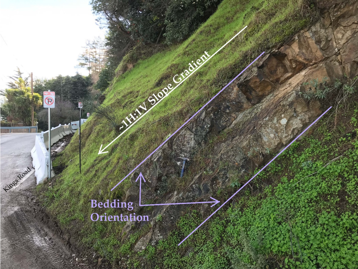
Figure 3: Photograph taken from Beatrice Road facing southeast towards Kings Road. In the fore-ground, fractured sandstone and shale bedrock of the Franciscan Complex is exposed on the slope. It appears that a previous rock-slope failure along a bedding plane (orientation annotated in purple) may have exposed this bedrock outcrop. Colluvial slopes are inclined at grades of approximately 100 percent (1H:1V Slope Gradient).
