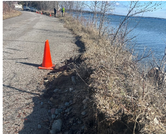
Figure 4: Shoreview Lane Damage – North Facing
