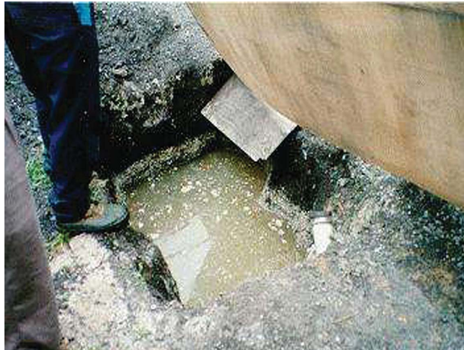
Figure 35: Failing septic tank.
