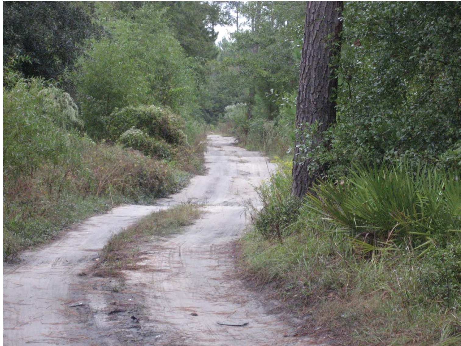
Figure 90: Unimproved dirt roads are difficult to maneuver, particularly for emergency vehicles.
