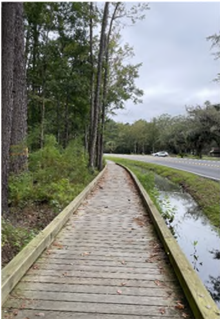
At the request of the residents, handrails were installed on this Buck Island Road boardwalk for additional safety.
