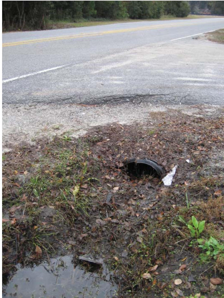
Figure 80: Typical clogged culvert found along the roadways.
