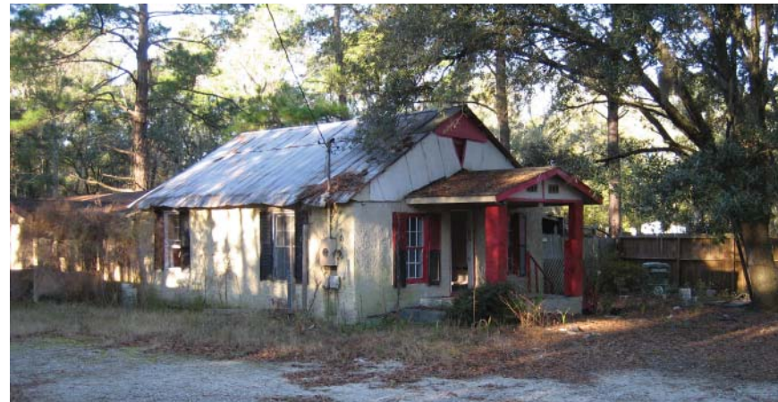
Figure 68: A condemned home in the BIS Neighborhood.
