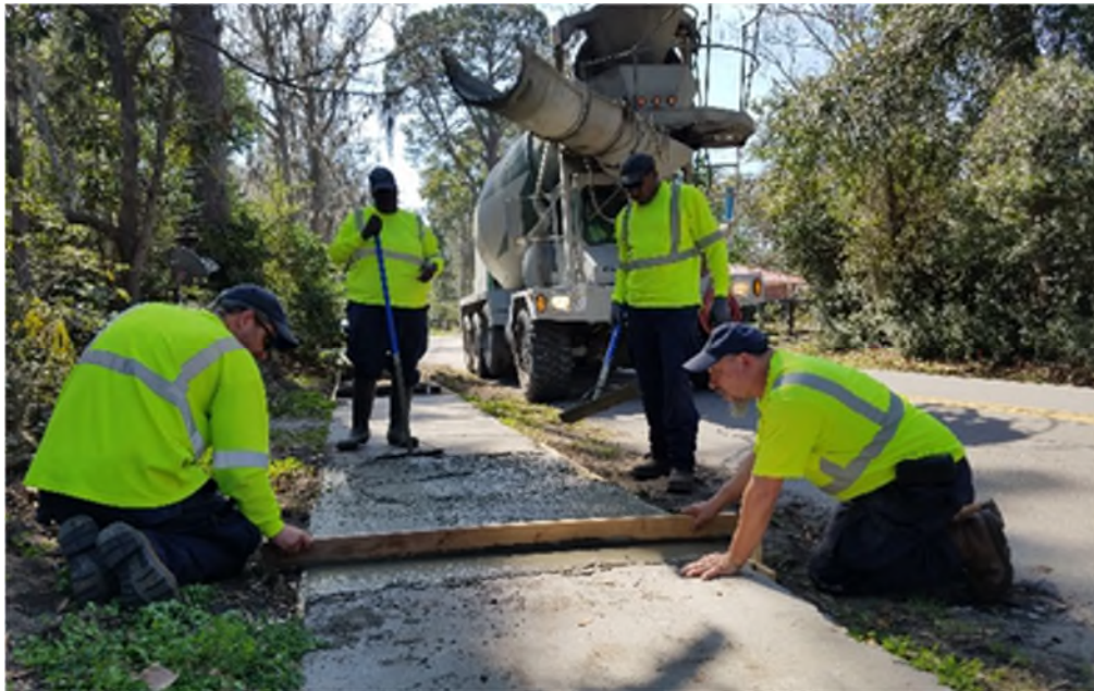
Approximately 2.65 miles of sidewalks have been installed in the Buck Island-Simmons ville neighborhood.
