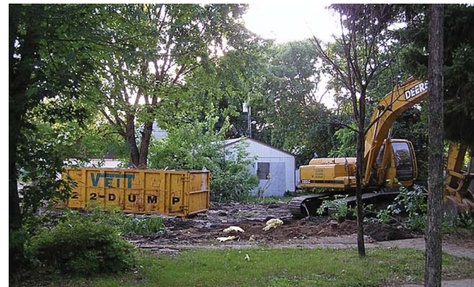
Figure 72: Demolition assistance can remove unsafe conditions from the Neighborhood, while also providing redevelopment opportunities for additional housing.
