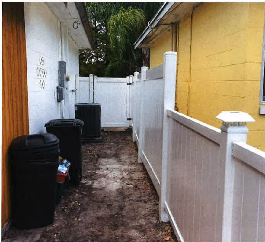
Photo 6: Electrical Services and Telecommunication wires hidden by 6ft high section.
