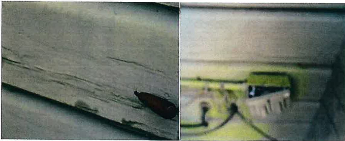
NORTH SIDE REAR severe rot on siding, (inserted 4" probe as seen). Also an open live electrical receptacle. Needs prompt attention. Paint is peeling in many places to bare wood allowing weather elements to penetrate the siding.
