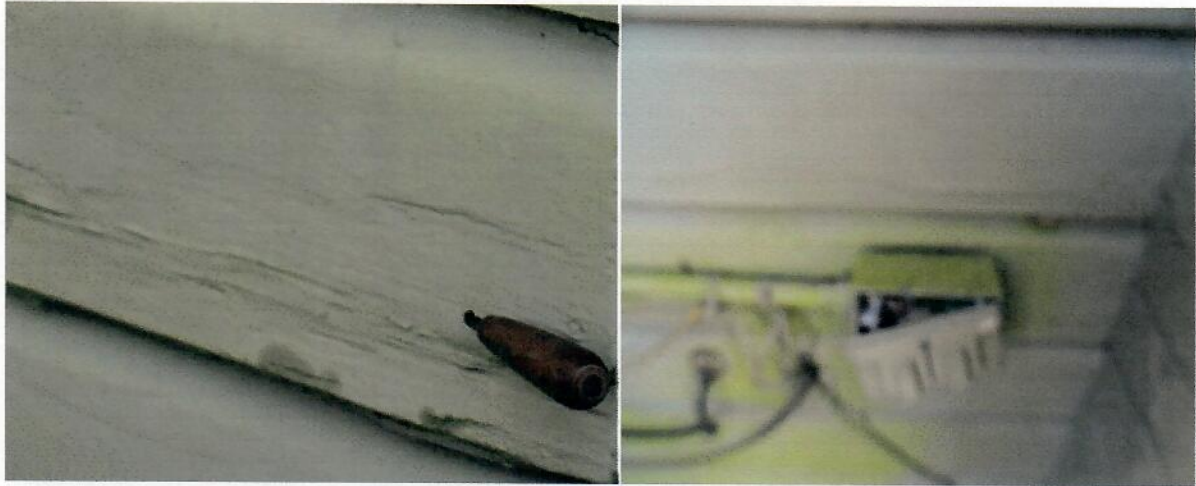
NORTH SIDE REAR severe rot on siding, (inserted 4" probe as seen). Also an open live electrical receptacle. Needs prompt attention. Paint is peeling in many places to bare wood allowing weather elements to penetrate the siding.
