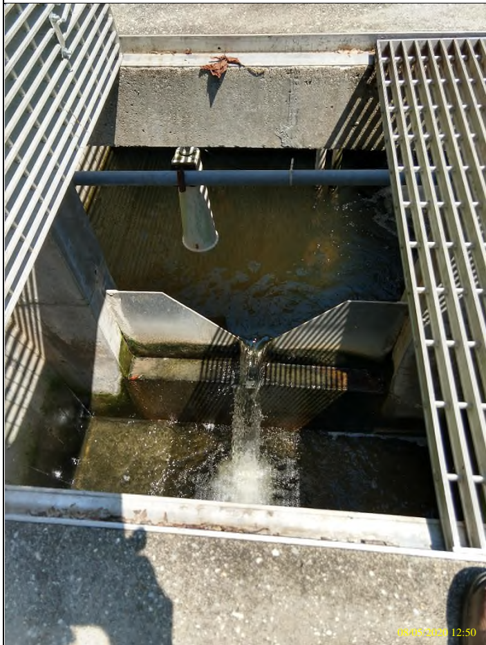
11) Final effluent sample collection point
