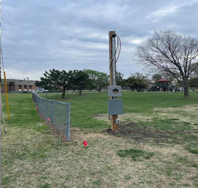
Bel Aire Park new electrical pole and sprinkler
