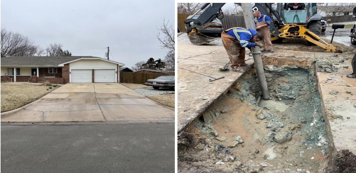
4335 Belmore water leak
