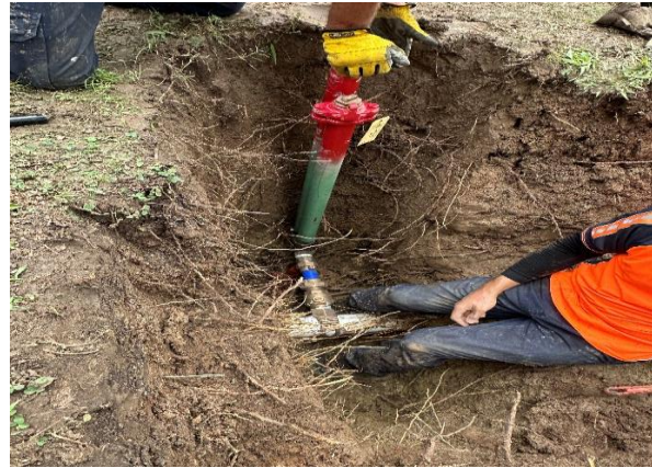
Flushing Hydrant Reck-
