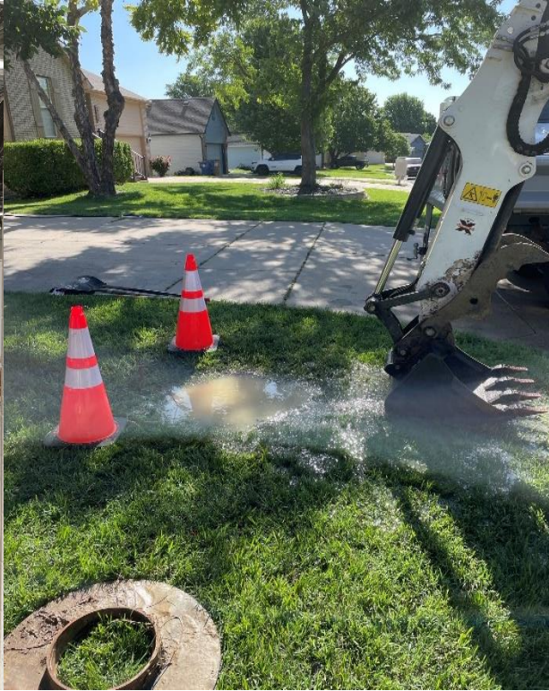
Water leak on main, St. James
