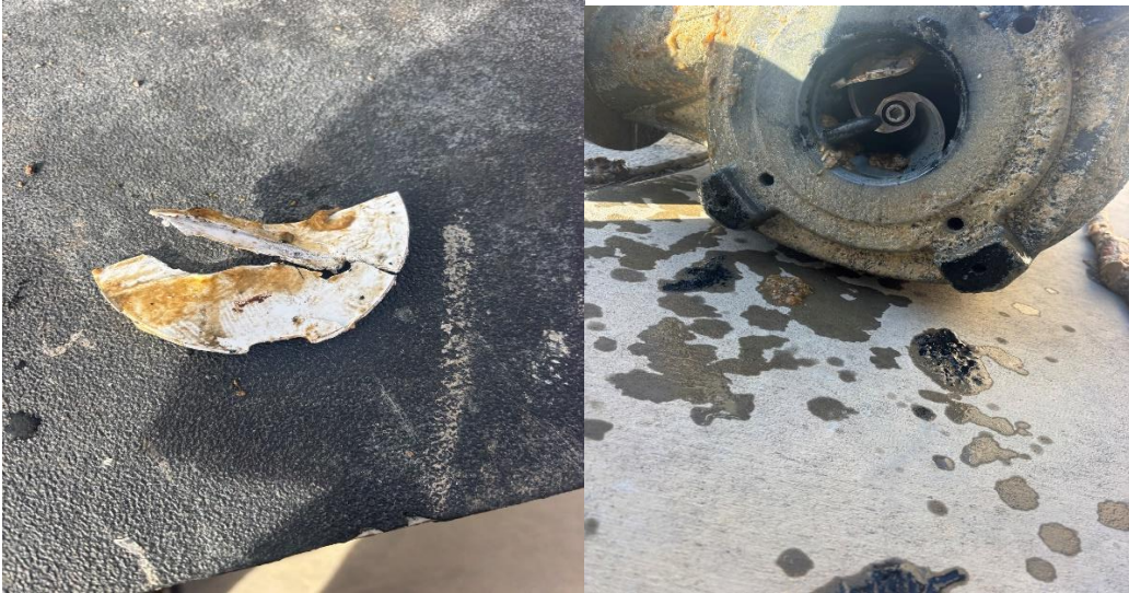
Oliver lift station pump failure due to plastic cap blocking the pump.
