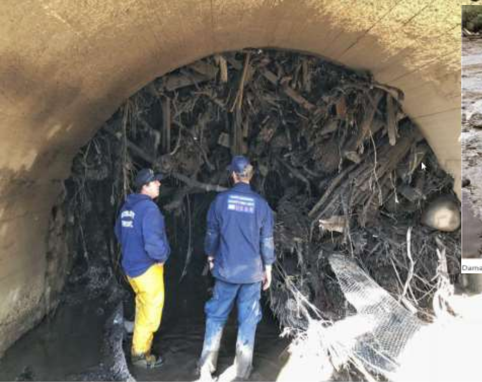
Firefighters look under a bridge at creek in Montecito that was jammed solid with debris from the deadly rains and mudflow January 9.
