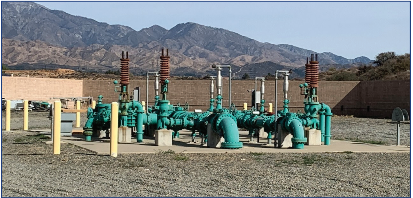
Above Grade Piping at Beaumont Mesa LS
