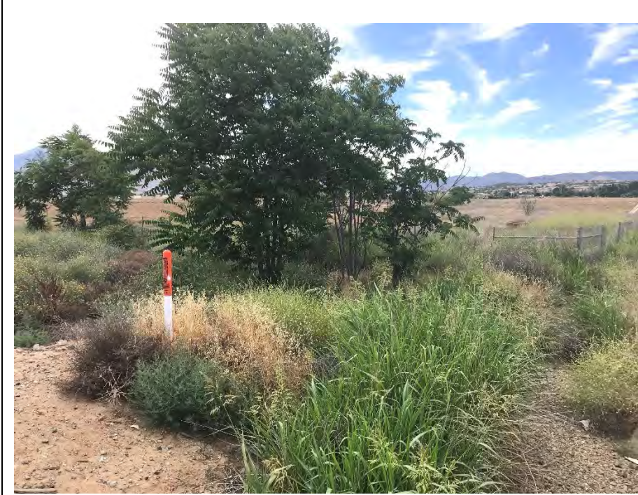
Photo 7 – Drainage A. Tree of Heaven and rushes/grasses growing near culvert
