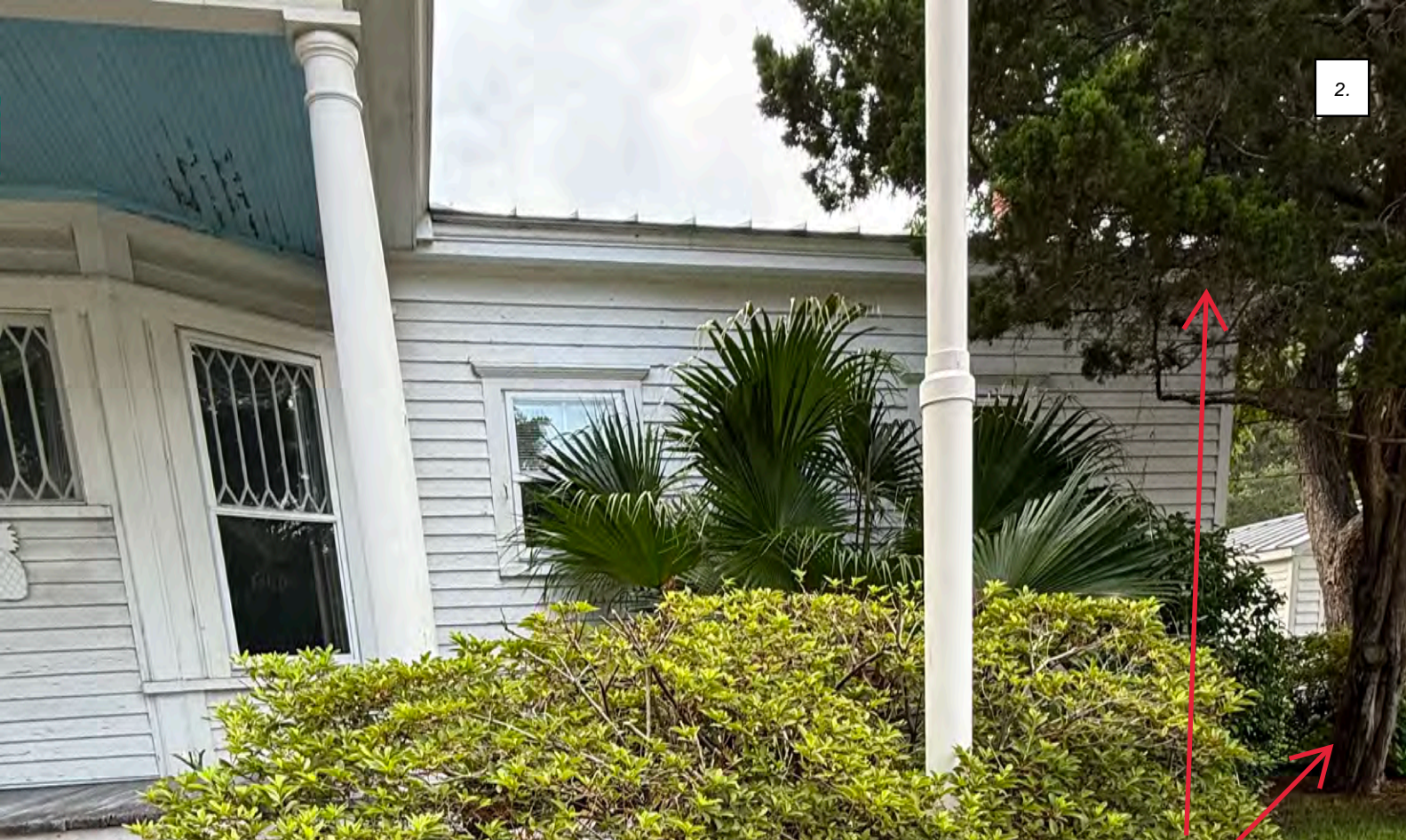
Remove cedar tree. Tree is located too close to the house. Tree roots are growing into the foundation and the branches are damaging the structure
