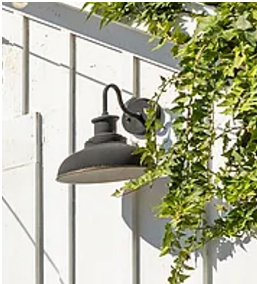
Existing Exterior Lights to remain
