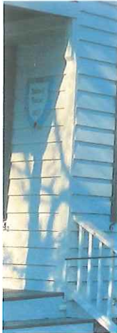
2x6 corner board faces toward the street to allow siding to end. Does not wrap corner.
