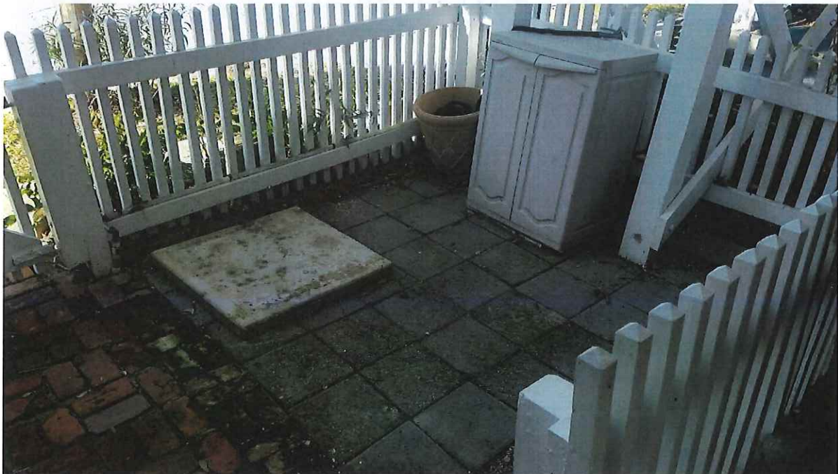
Existing gray paving stones to be removed and replaced with period correct reclaimed brick.
