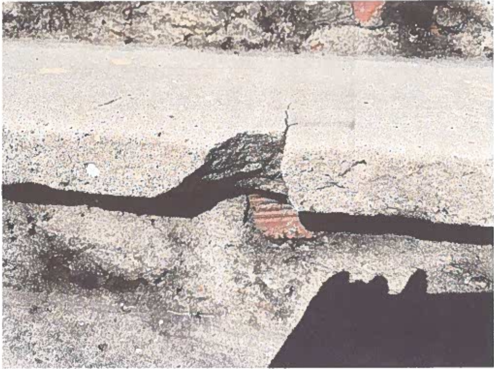
Some steps have portions missing from wear and tear
