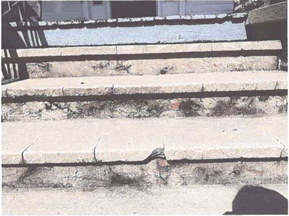
More detail of step deterioration
