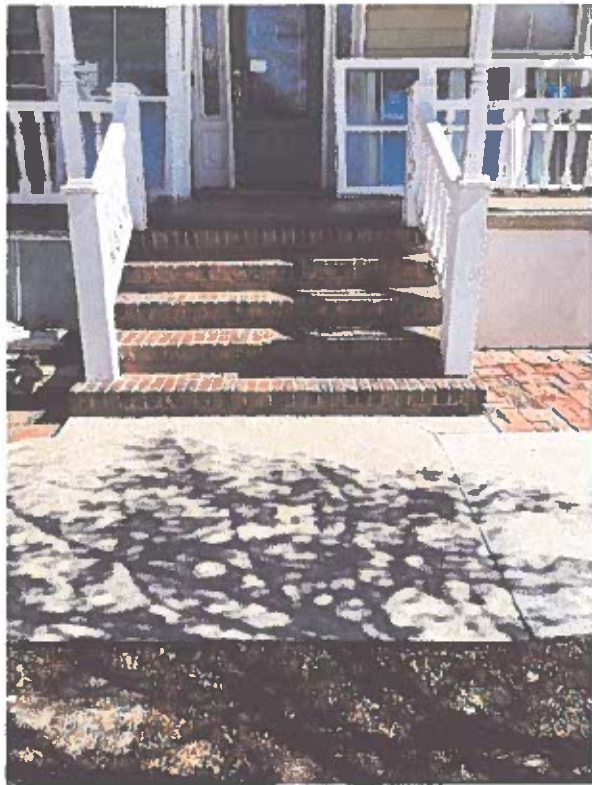
This is the steps and walkway at 120 Craven
