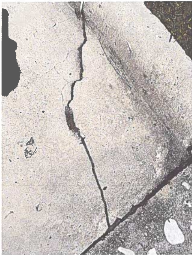
Detail of more cracking at the front of the walk
