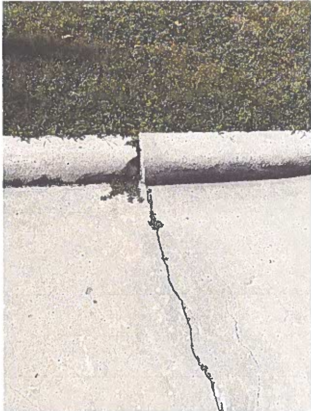
The concrete molding is also deteriorating
