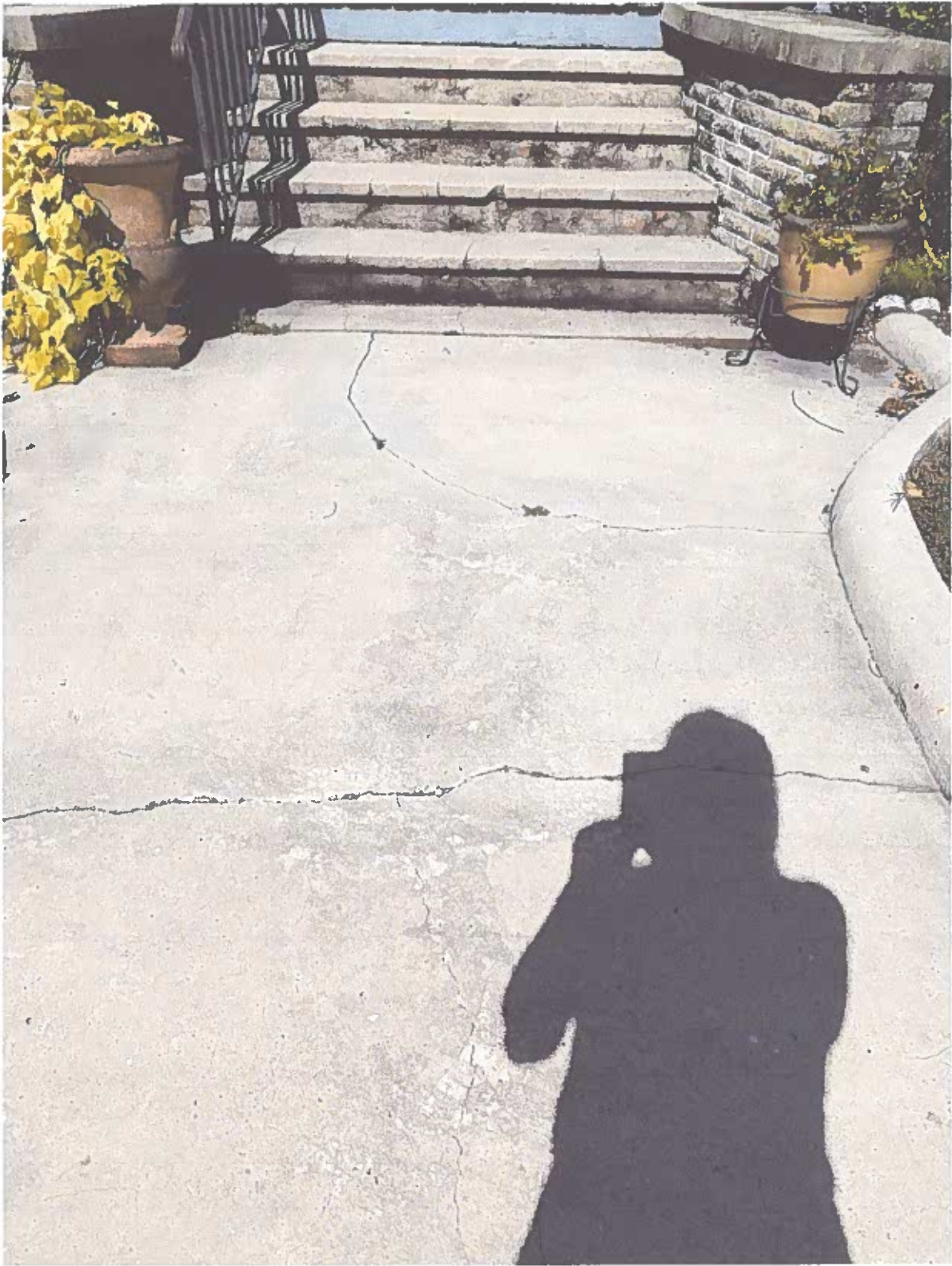
Walkway is becoming a tripping hazard and water pools at the lower step due to subsidence of the walk
