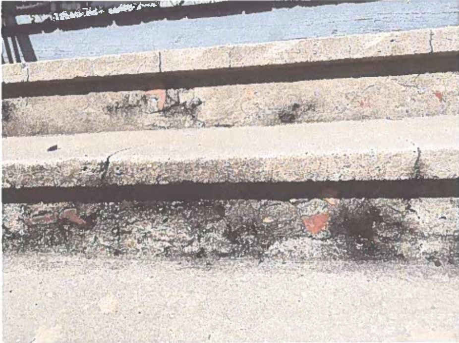
Detail of brick construction showing the cracking in the step
