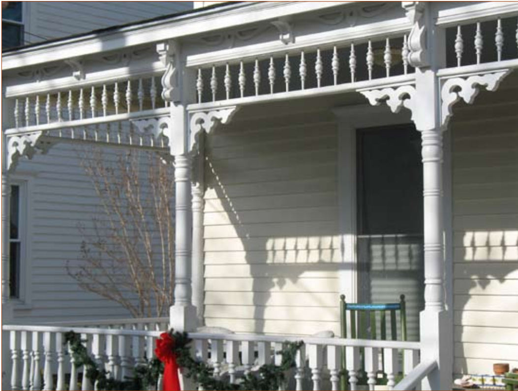
Character-defining features of this late 19 th -century Queen Anne style porch in Beaufort include the turned posts and pilasters, the turned balustrade, the jig-sawn brackets, and the row of spindles below the eaves.
