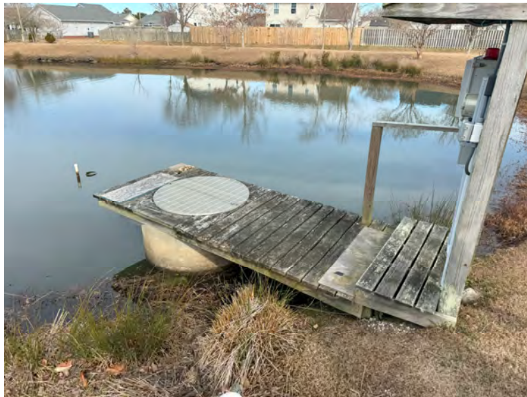
Photo 3. Meeting Street retention pond pump station (Photo taken by WKD Staff 02/08/24).
