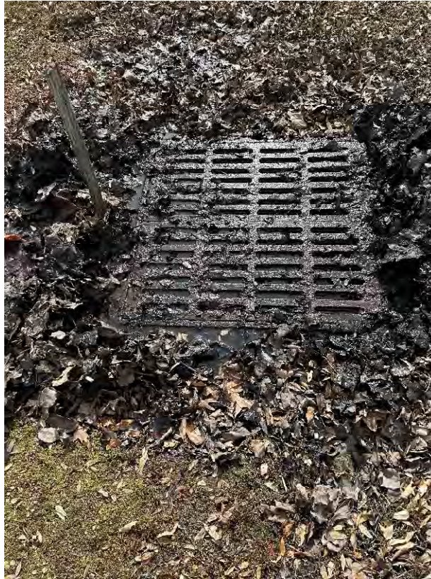
Photo 4. Drop inlet grate just upstream of the pump pond filled to the rim in non-flooding conditions (Photo taken by WKD Staff 02/08/24).
