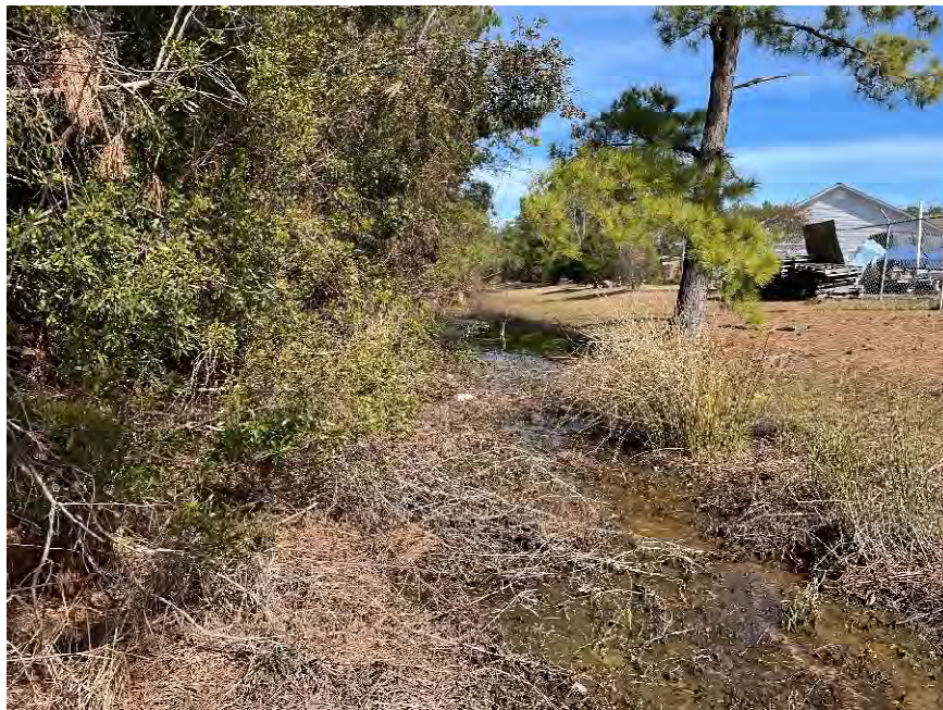
Photo 5. Meeting Street drainage ditch looking downstream toward northern outfall (Photo Taken by WKD Staff 02/08/24).
