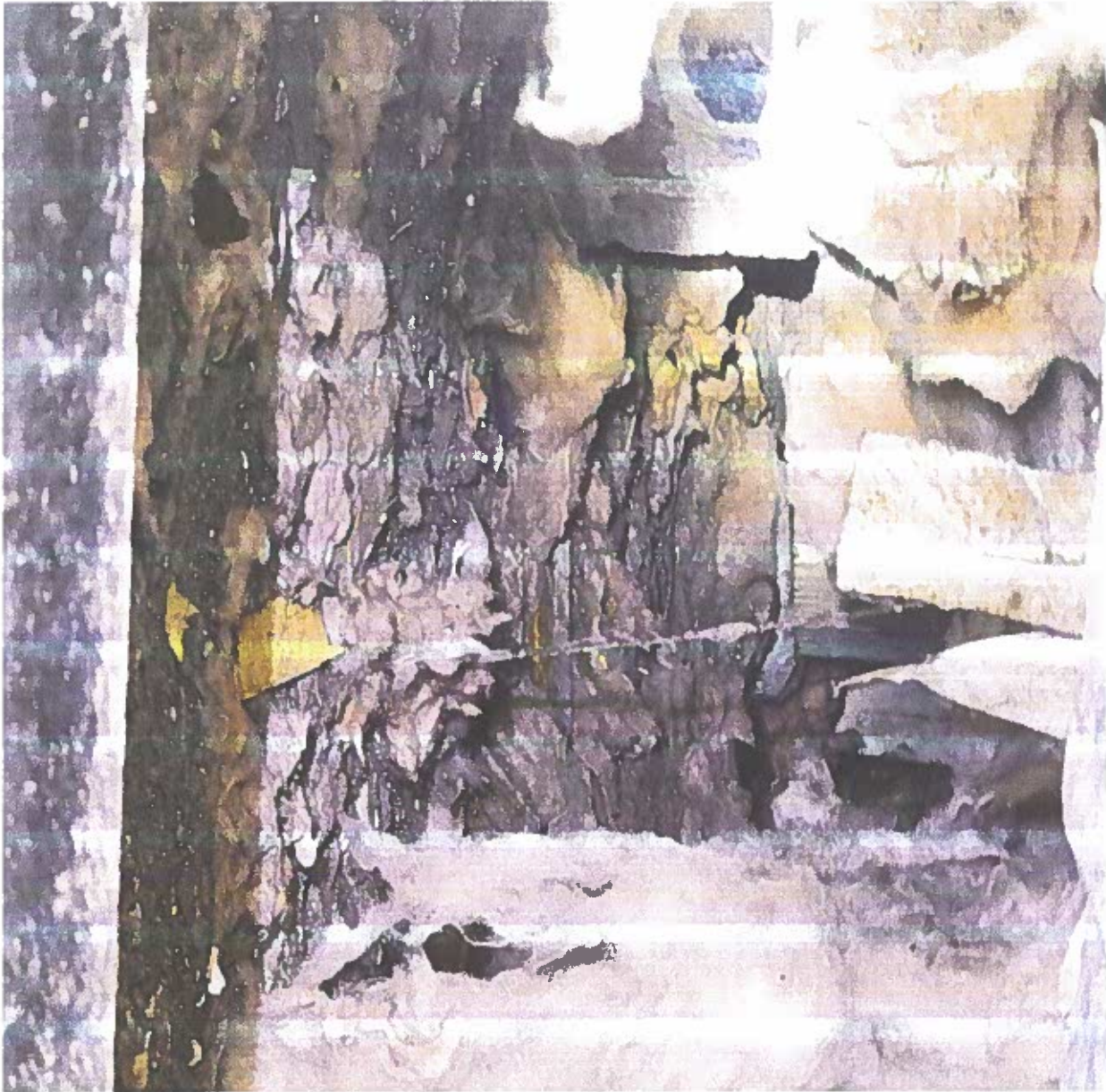
Temporary 4x4 on concrete block and eroded mortar in brick pier
