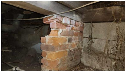
Spalling brick support piers
