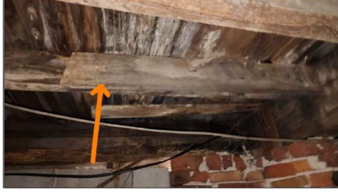
Floor joists too far apart to adequately support subfloors resulting in improper patchwork to prevent deflection
