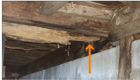
Completely deteriorated support beams and floor joists due to moisture and insect related damage
