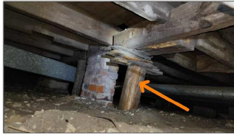
Irregular support logs and wood shims improperly holding support beams with no concrete base foundation; not up to code
