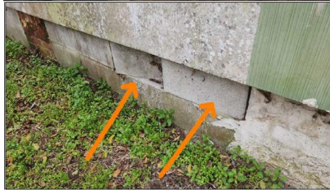
Deteriorated brick and grout; shifting concrete support blocks
