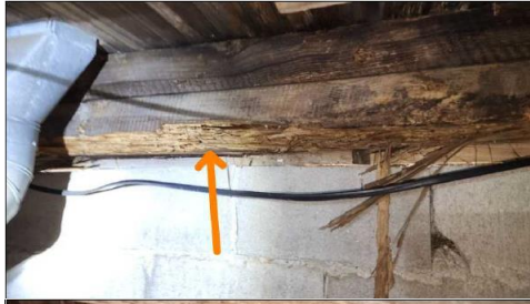
Completely deteriorated support beams and floor joists due to moisture and insect related damage
