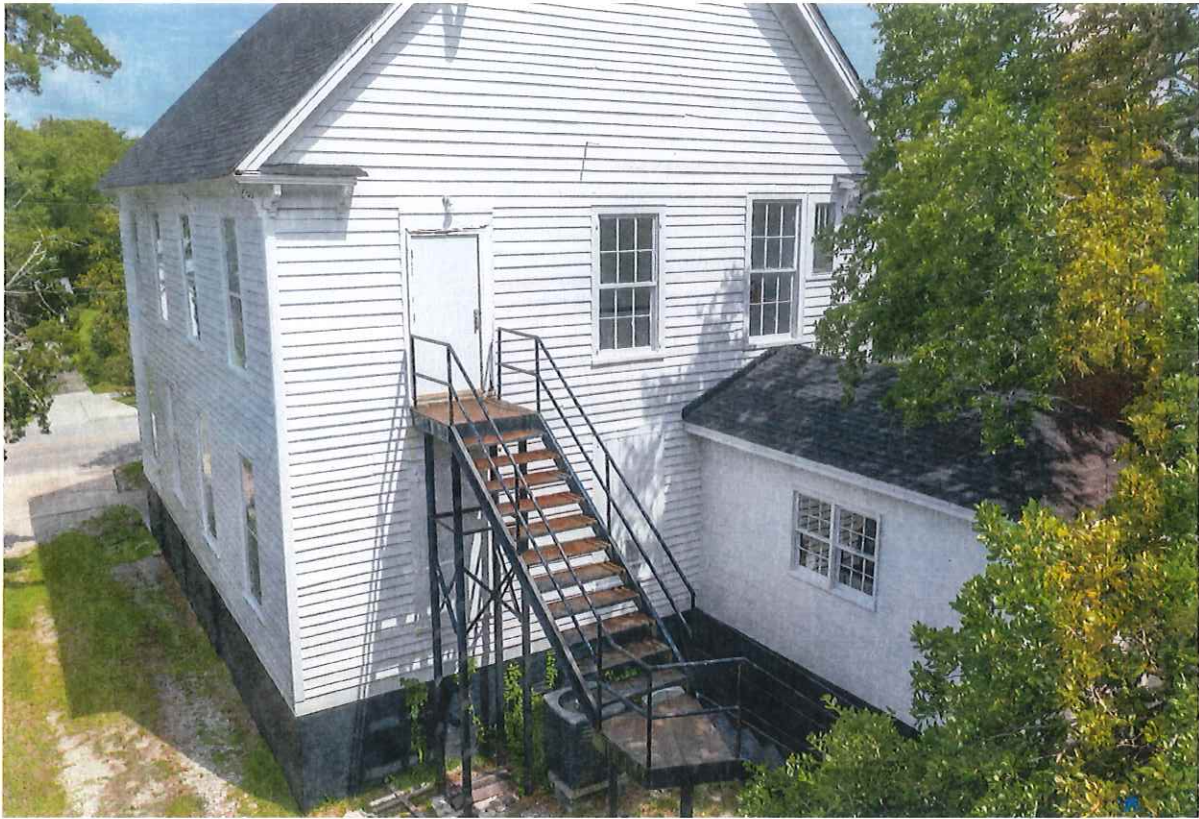
View of East facade. Entire structure to be extended approximately 64 feet, requiring the removal of metal stairs, and removal of kitchen addition on rear. Utility equipment to be relocated; location TBD.
