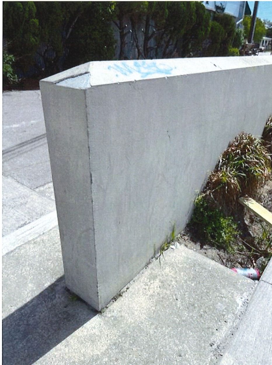
Existing Site Wall; CMU with smooth parge coat; Proposed perimeter seat wall to match; Top of wall proposed to be flat; Color to match existing structure. Option#1
