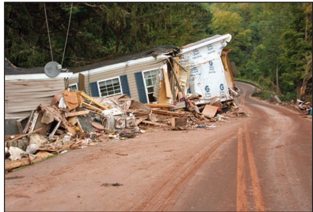
A flooded manufactured home can float off its foundation and cause additional damage nearby.
