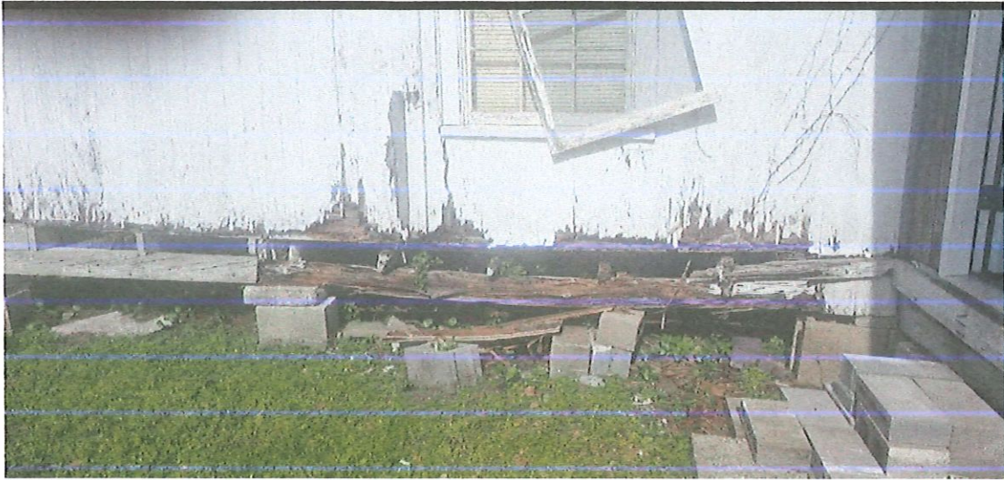
Photo 032625 deterioration of foundation and horizontal beam
