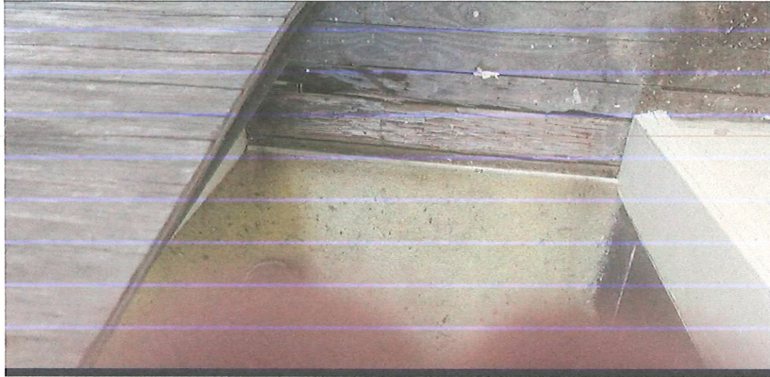
Photo 032625 deterioration of flooring
