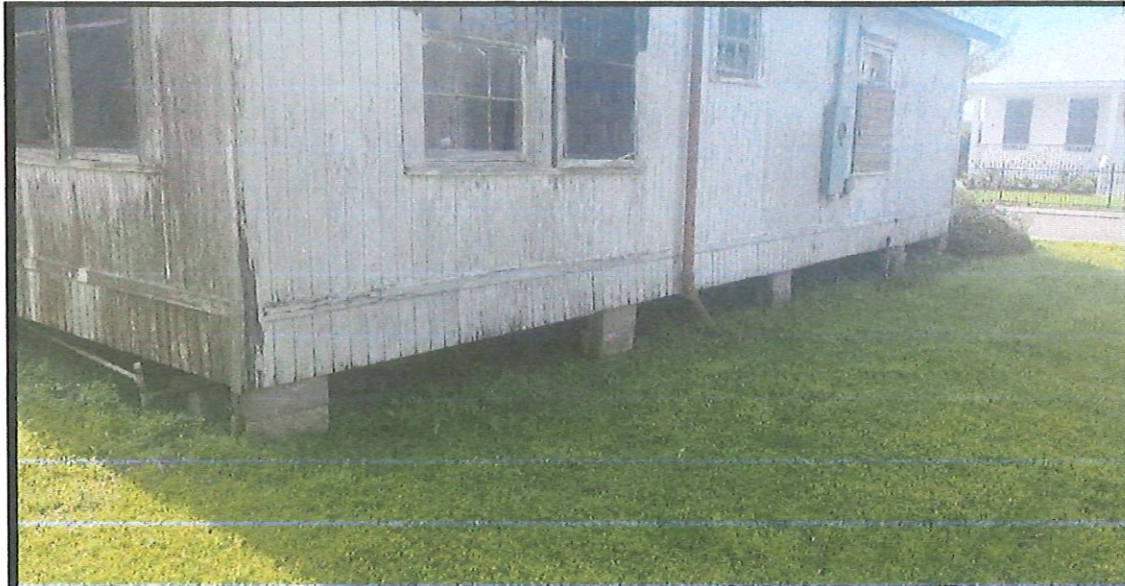
Photo 032625 unevenness of cinder blocks supporting structure
