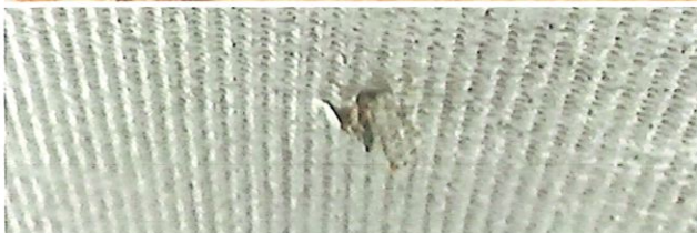
Roofing nails piercing roof decking
