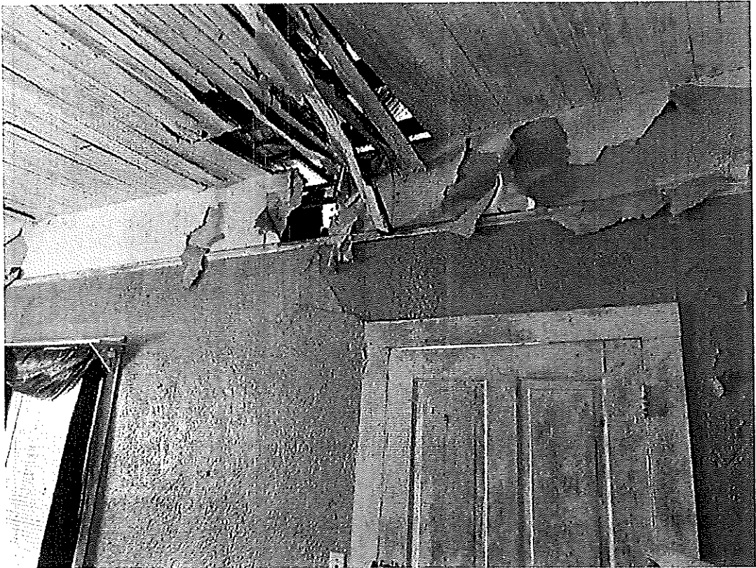
Photo 092023 interior mold and structural cracks above door indicating settlement.
