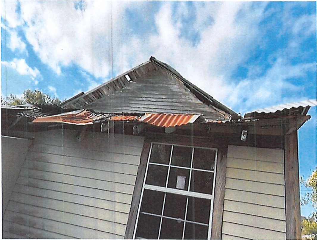
Photo 092023 a non existent load path from roof to exterior walls and indications of settlement. Sincerely
