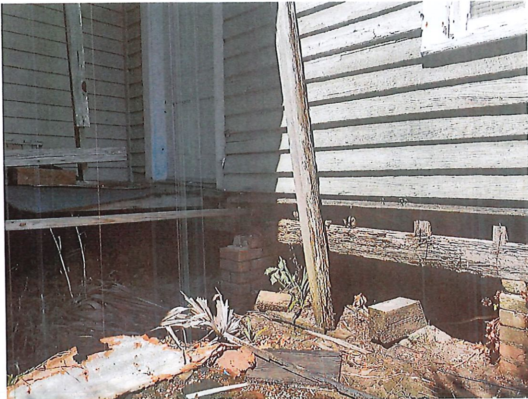
Photo 091223 deterioration from weathering and termites of horizontal support beam
