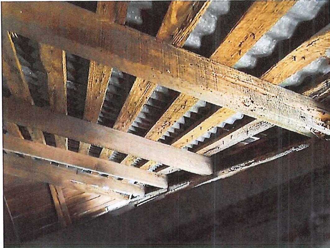
Photo 091223 rafter and purlin damage and a non-existent load path from the roof to the exterior walls
