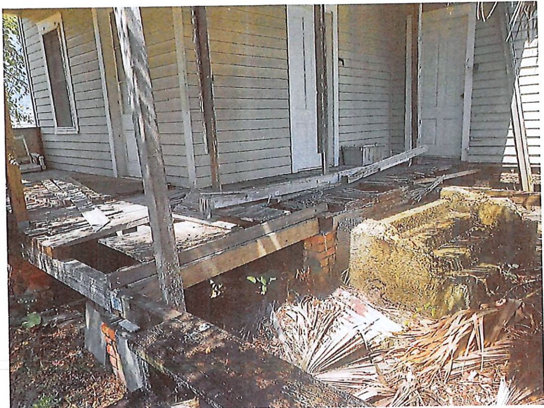
Photo 091223 deterioration of foundation elements
