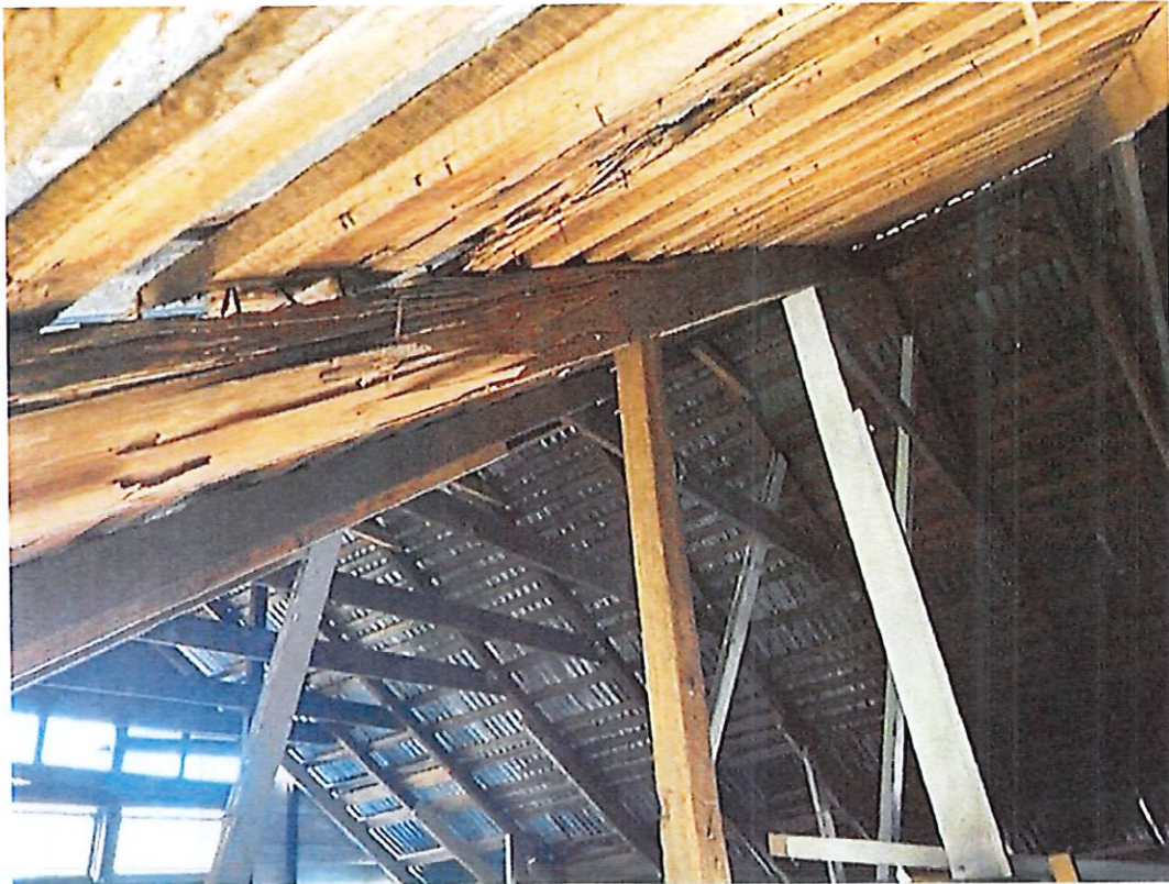
Photo 092023 roof deterioration of purlins, rafters, and cross bracing. In addition, no indication of a load path connecting rafters and plates to walls.
