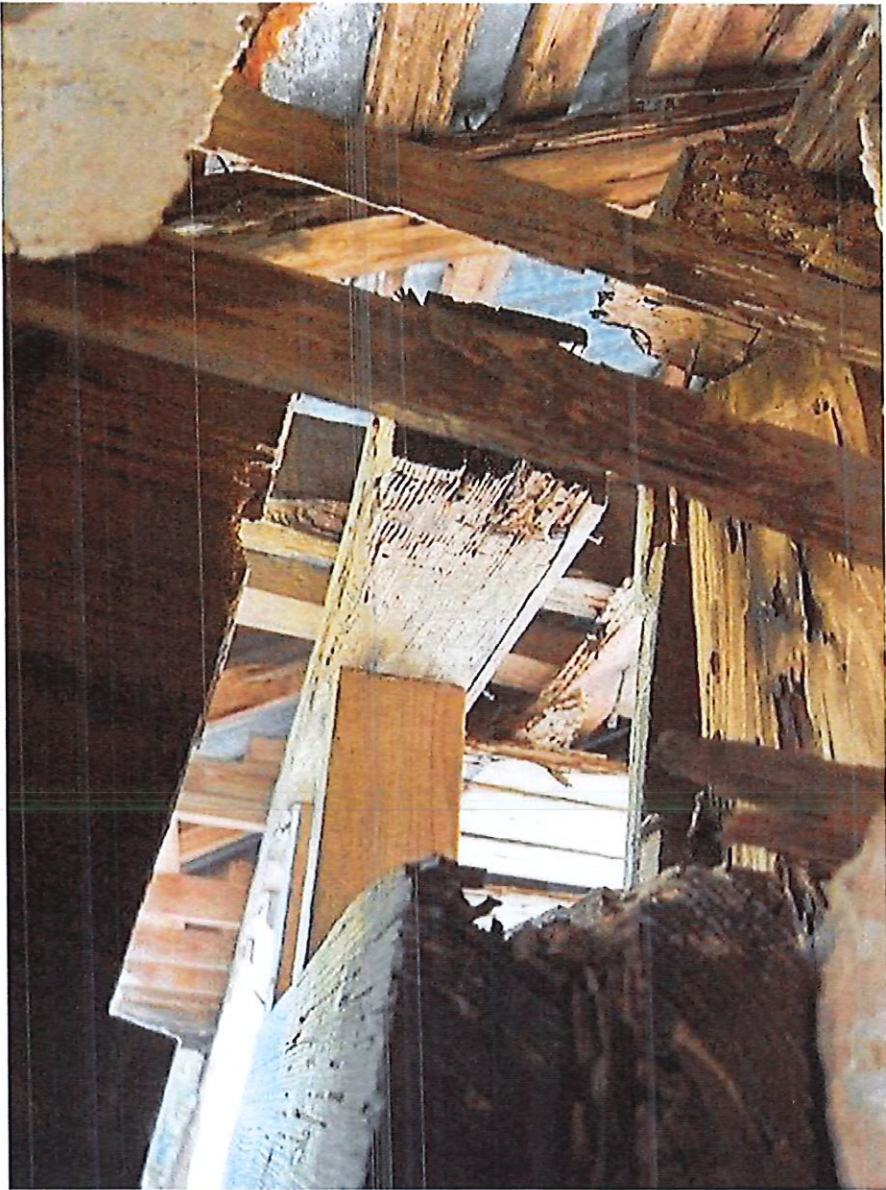
Photo 092023 roof deterioration from weathering and termites of rafters, cross bracing and purlins
