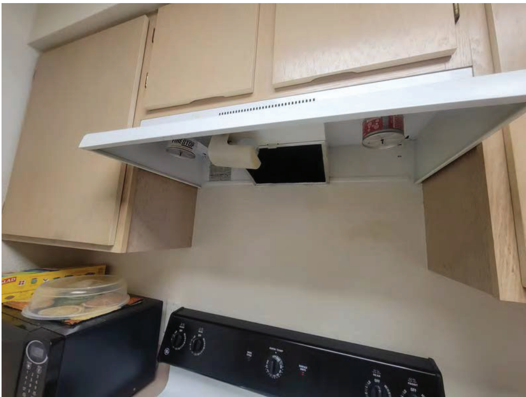
146. Typical unit range hood
