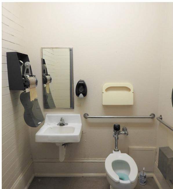
Photo 13: Existing non-ADA compliant 1 st floor restroom.
