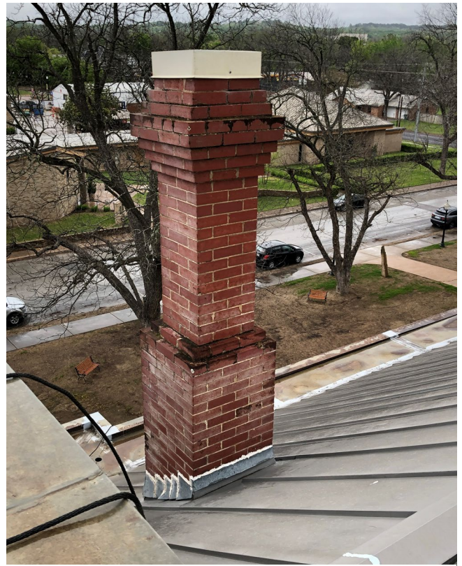
Photo 4: Existing sheet metal roofing to be replaced with slate roofing. Brick chimneys will be repointed 100%
