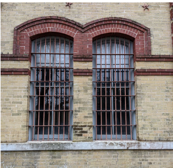
Photo 9: Windows and window grilles to be restored 100%. Masonry restoration includes selective brick repairs/replacement, repointing
