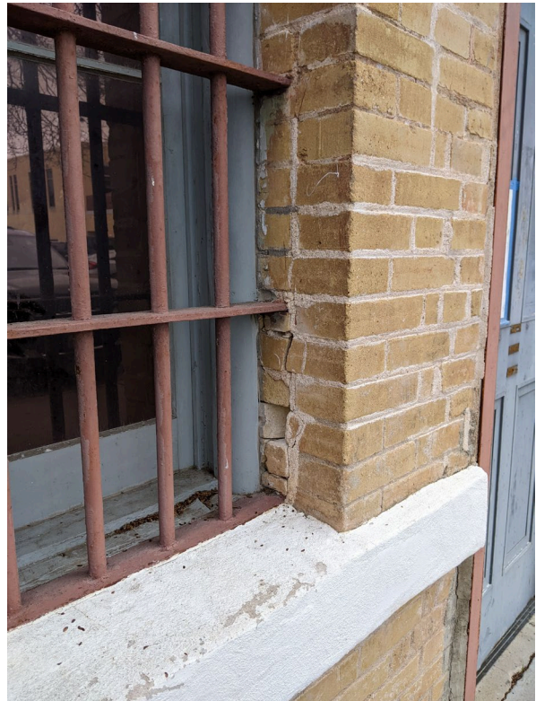
Photo 8: Parge coat to be restored 100%. Masonry restoration includes selective brick repairs/replacement, repointing 100%.
