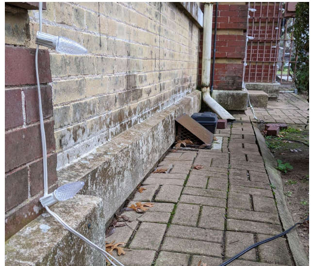
Photo 6: Existing brick pavers and covered crawlspace ventilation. Perimeter of building will receive 2' wide concrete mow strip.
