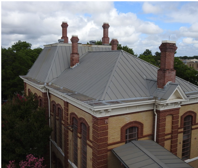
Photo 5: Existing sheet metal roofing to be replaced with slate roofing. Brick chimneys will be repointed 100%
