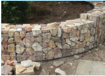
STORMWATER COLLECTION OVERFLOW BLOCKS / GABIONS
